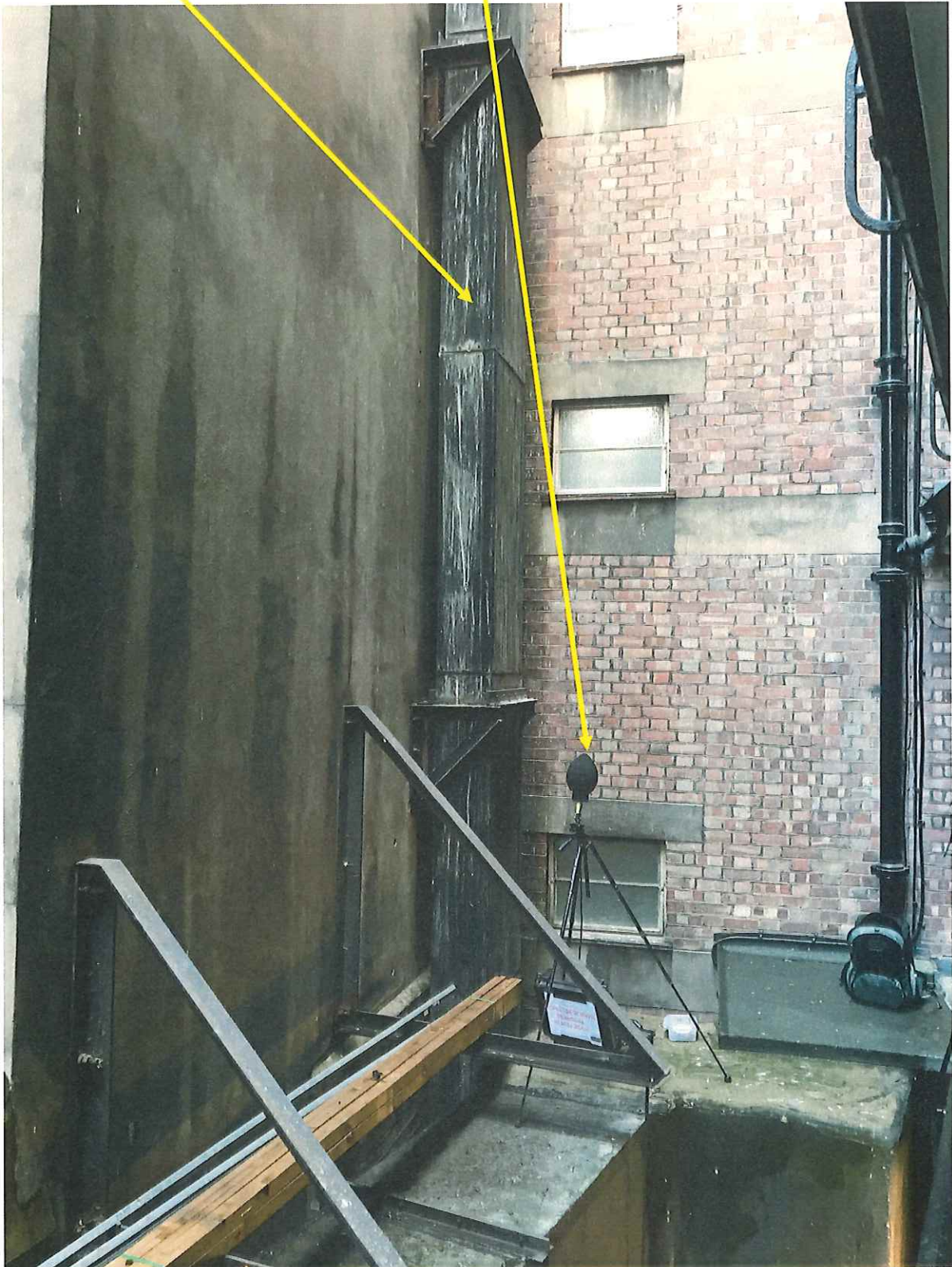
Photo F – Location of microphone at low level next to basement extract ducting
