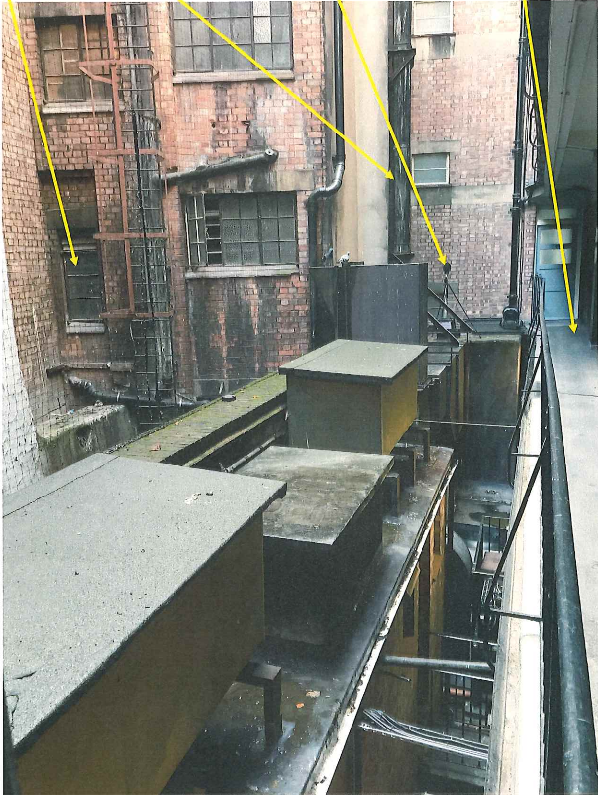
Photo C – Bottom of Light Well Behind the Residential Flats in Phoenix House
