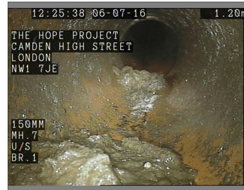
Photo: 19_19_120_A.JPG 1.2m, Settled deposits, coarse, 10% cross-sectional area loss
