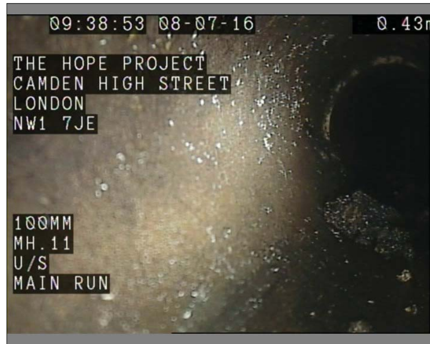
Photo: 27_27_178_A.JPG 0.43m, Settled deposits, coarse, 10% cross-sectional area loss
