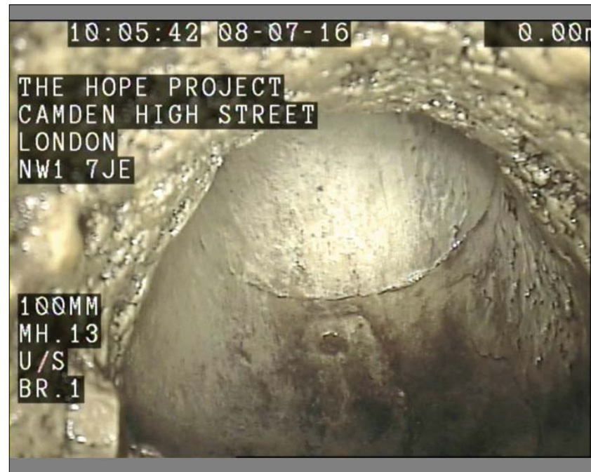
Photo: 29_29_193_A.JPG 0m, Attached deposits, encrustation, from 9 to 2 o'clock, 10% cross-sectional area loss
