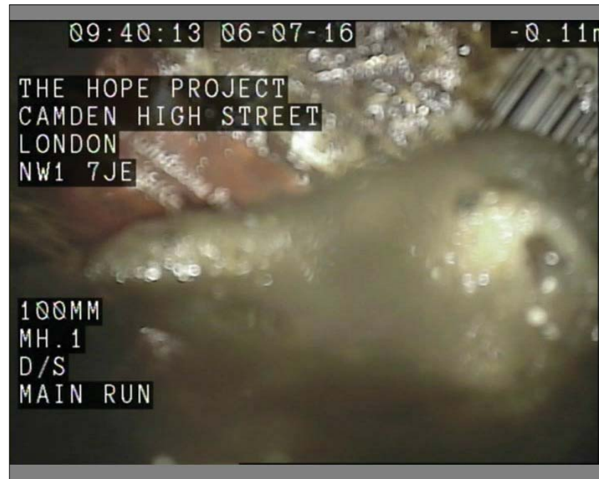
Photo: 6_6_21_A.JPG 0.11m, Settled deposits, fine, 80% cross-sectional area loss
