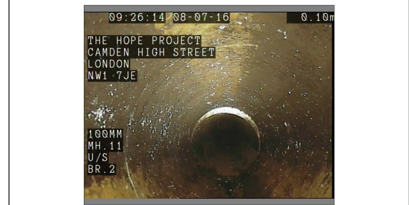
Photo: 26_26_162_A.JPG 0.1m, Crack, circumferential, from 7 to 12 o'clock
