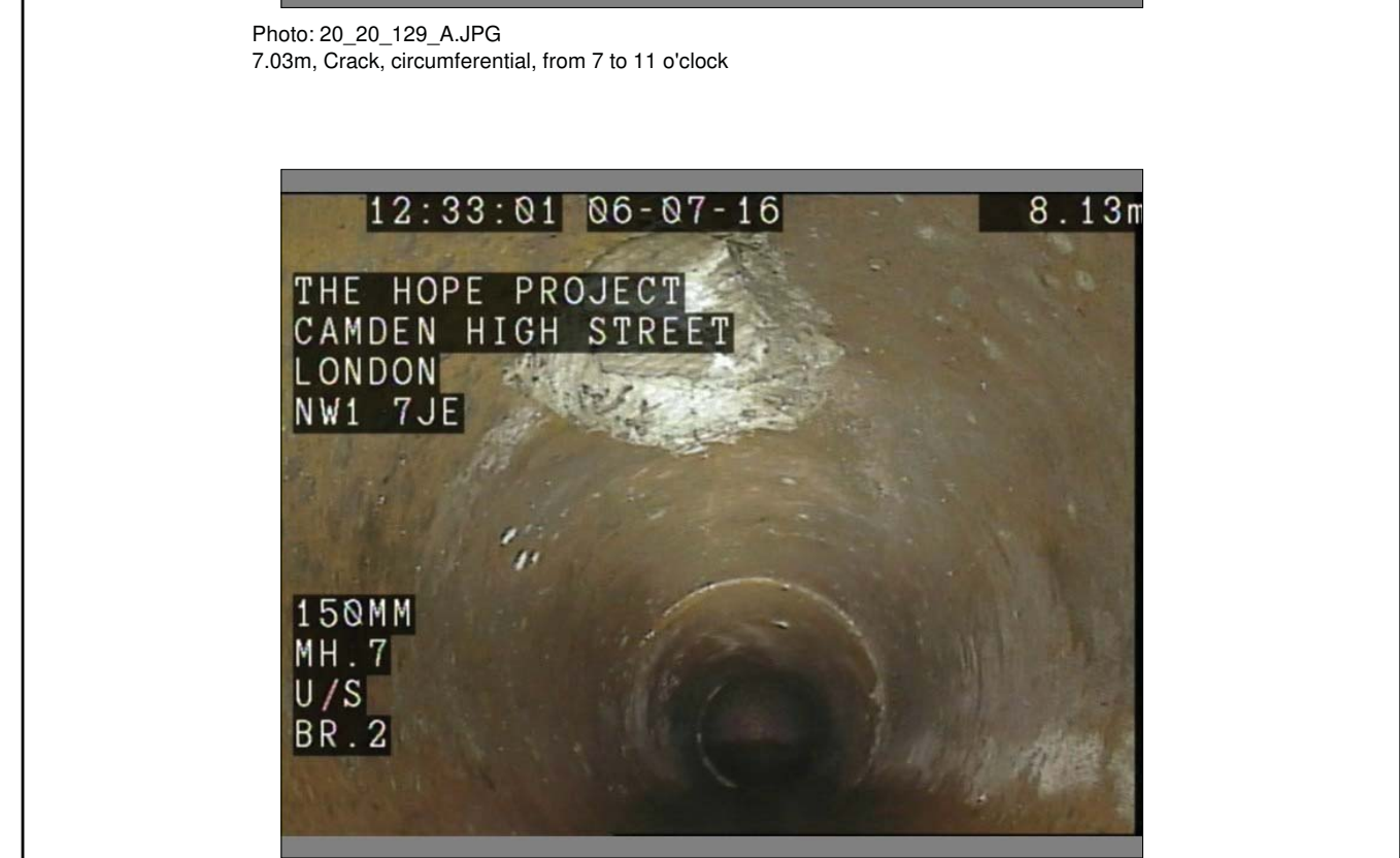
Photo: 20_20_131_A.JPG 8.13m, Broken pipe, from 10 to 12 o'clock
