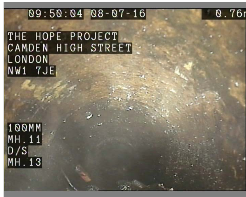
Photo: 28_28_187_A.JPG 0.98m, Settled deposits, coarse, 10% cross-sectional area loss
