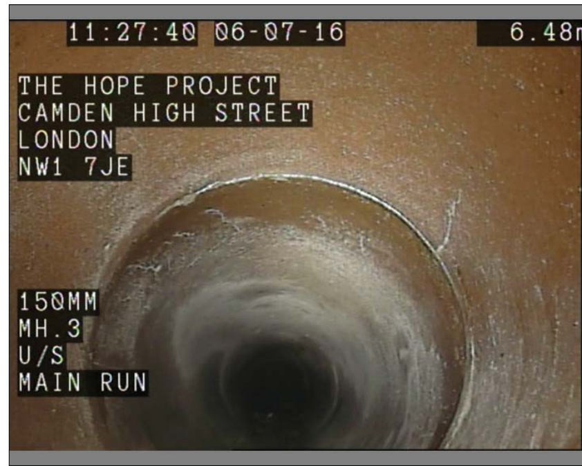
Photo: 12_1_9_18072016_124627_A.jpg 6.48m, Crack, longitudinal at joint, at 2 o'clock
