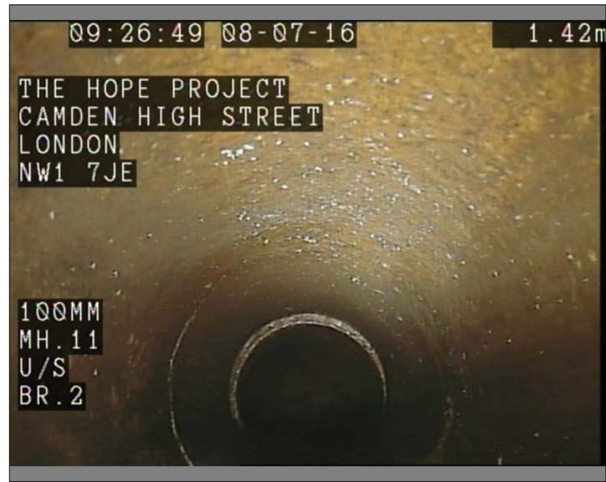
Photo: 26_26_163_A.JPG 1.42m, Crack, circumferential, from 7 to 5 o'clock
