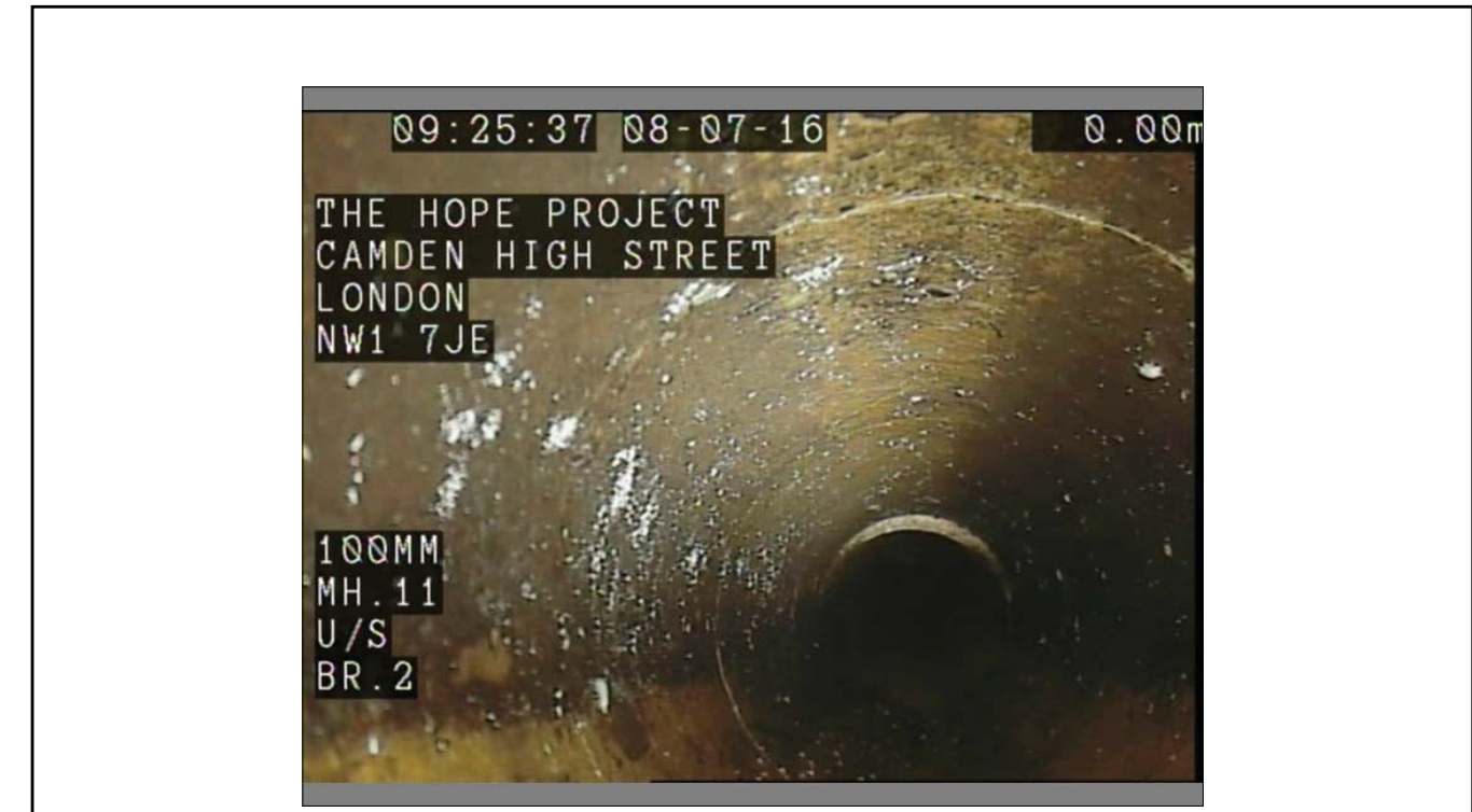
Photo: 26_26_161_A.JPG 0m, Crack, circumferential, from 7 to 4 o'clock
