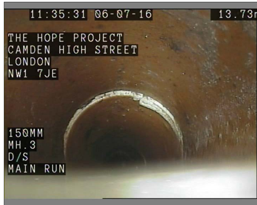
Photo: 14_14_82_A.JPG 13.84m, Broken pipe at joint, from 1 to 3 o'clock
