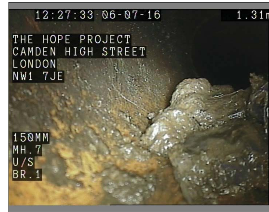
Photo: 19_19_121_A.JPG 1.31m, Settled deposits, coarse, 10% cross-sectional area loss
