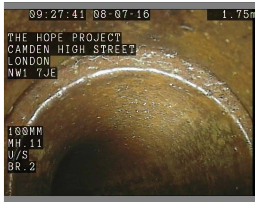
Photo: 26_26_164_A.JPG 1.75m, Crack, circumferential at joint, from 7 to 3 o'clock
