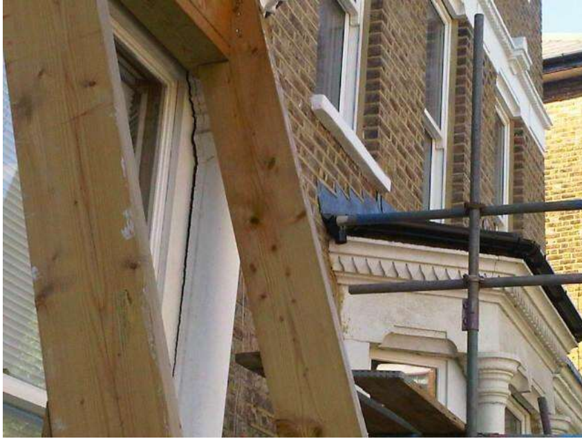
Cracked window frame and emergency structural support at 92 South Hill Park, caused by basement development next door
