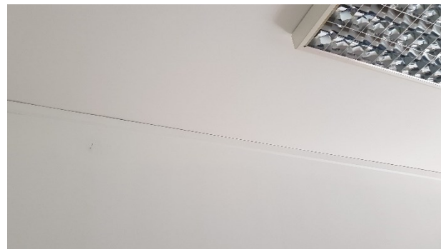
Fig. 18 – Existing white plastic trunking in academic office, running along wall/ceiling join
