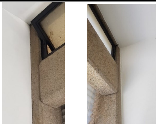
Fig. 17 – Existing joints where partition wall meets concrete superstructure (exposed concrete sections to be carefully treated to remove traces of the partition from the exposed aggregate).
