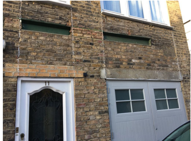
Differing brickwork, steelwork & concrete
