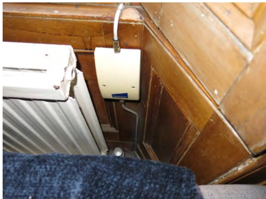
Figure 10: View of the window recess with radiator and sofa along the bottom edge of the picture
