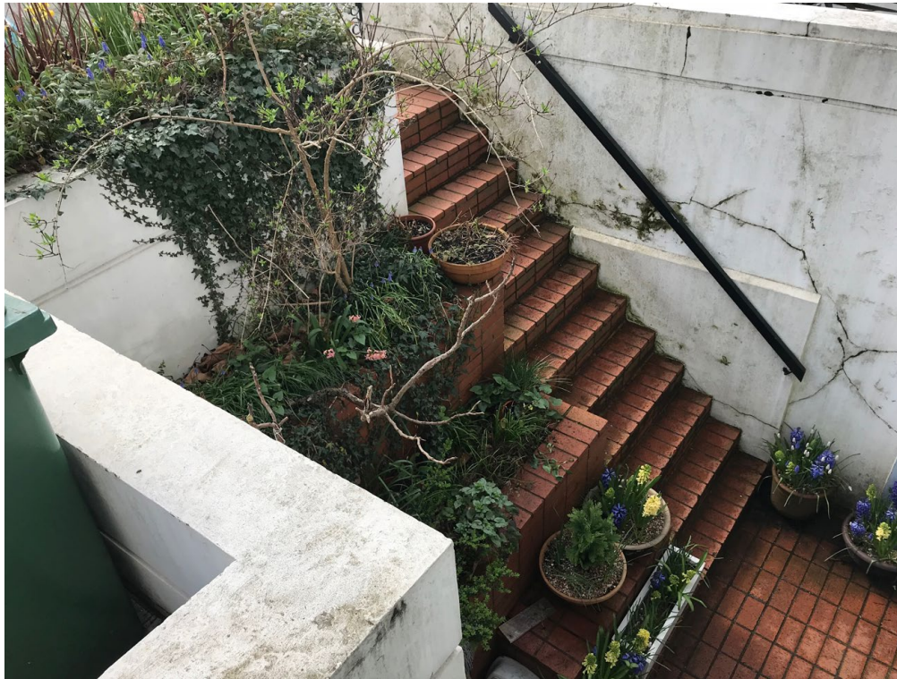
Fig. 12: The tiered planters and basement staircase, as viewed from the ground floor entrance path
