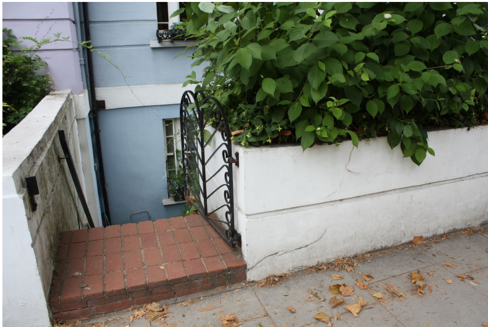
Fig. 8: The basement entrance viewed from Regent's Park Road, showing the step up from street level and existing boundary wall
