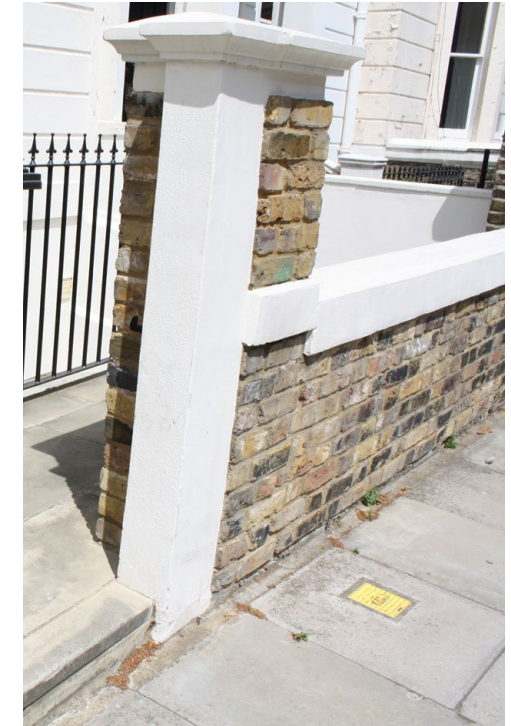
Fig. 21: The render and brick pier to 2 St. Mark's Terrace, featuring a paved front garden and metal railings. This style of front garden is typical throughout the Conservation Area
