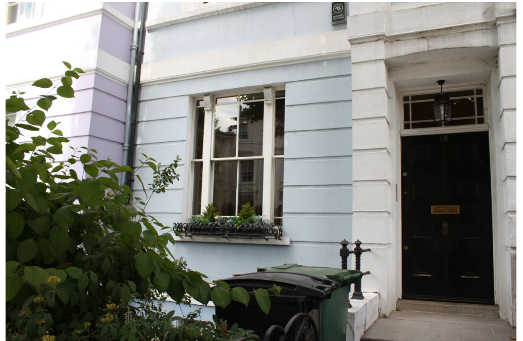
Fig. 11: The front elevation of the ground floor entrance, and existing sash window to be remade
