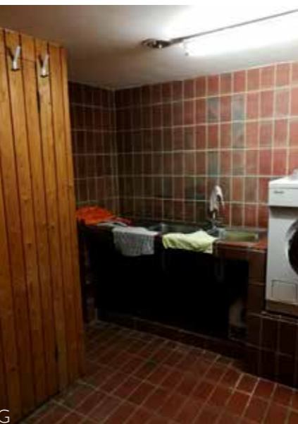
Photos D-G These photos show boxing in to the original lightwell windows as well as the remains of an original arch to the kitchen hearth which now holds a new boiler. Photo G shows the utility area to the back of the basement.
