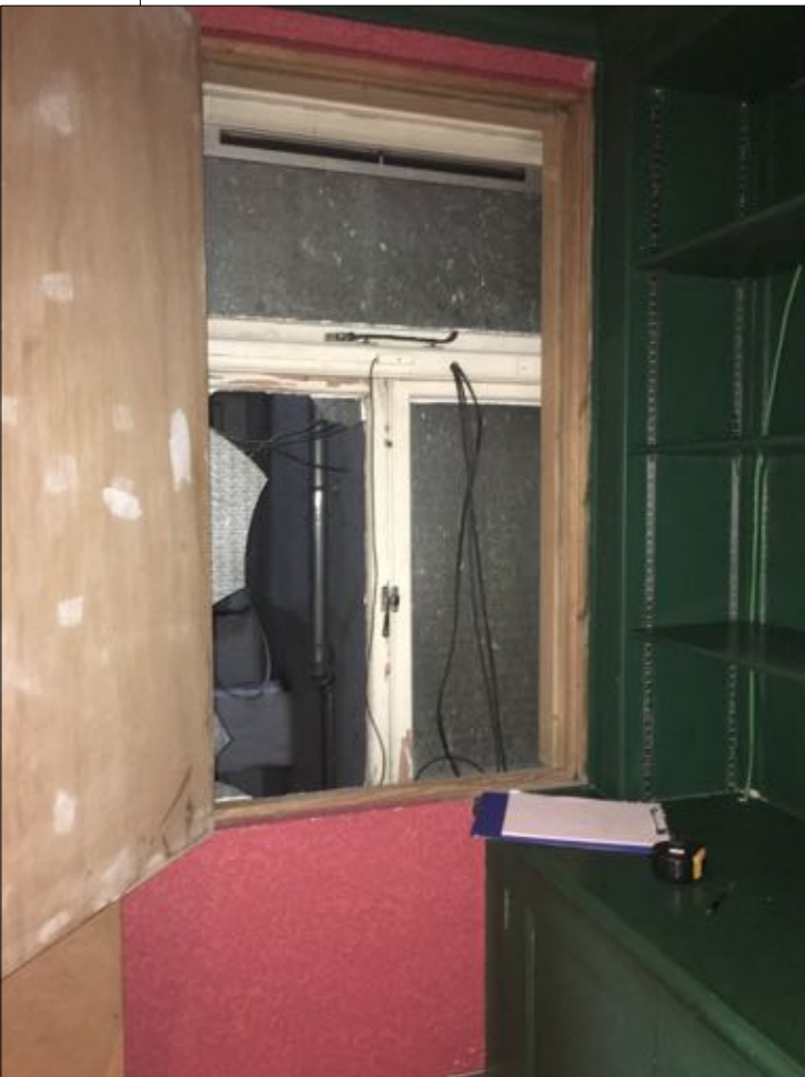
windows to be repaired and overhauled
