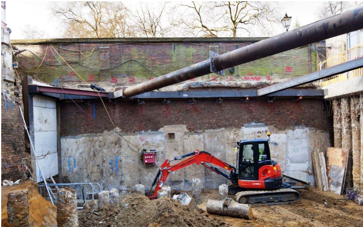
Photo 5 “Tudor” red brick perimeter wall [13] sandwiched between lower concrete underpinning and 19th-century rebuilt perimeter wall above modern ground level (note also natural sand and clay bottom left).
