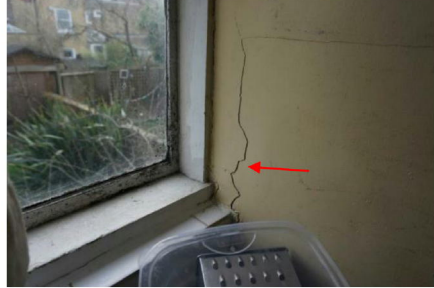
30B – Kitchen – Vertical Crack
