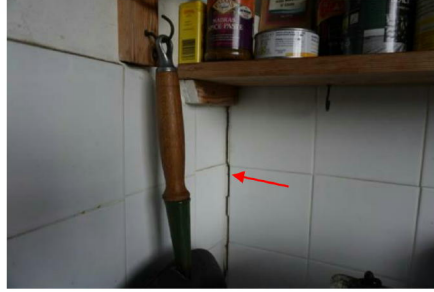
30C – Kitchen – Vertical Crack at Junction
