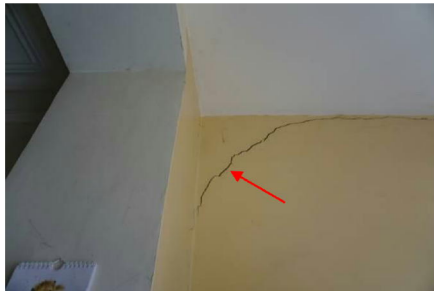
30B – Kitchen – Diagonal Crack to Left Wall
