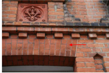
Front Elevation – Crack above entrance porch (not subsidence)
