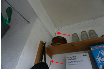
30C – Kitchen – Vertical Crack at junction
