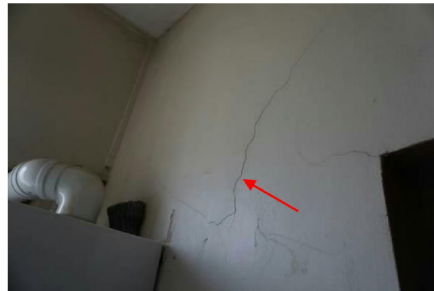
30B – Utility Room – Diagonal Crack to Right Wall
