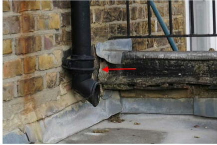
View of Rear Projection Roof – Separation of Parapet from rear elevation of main house
