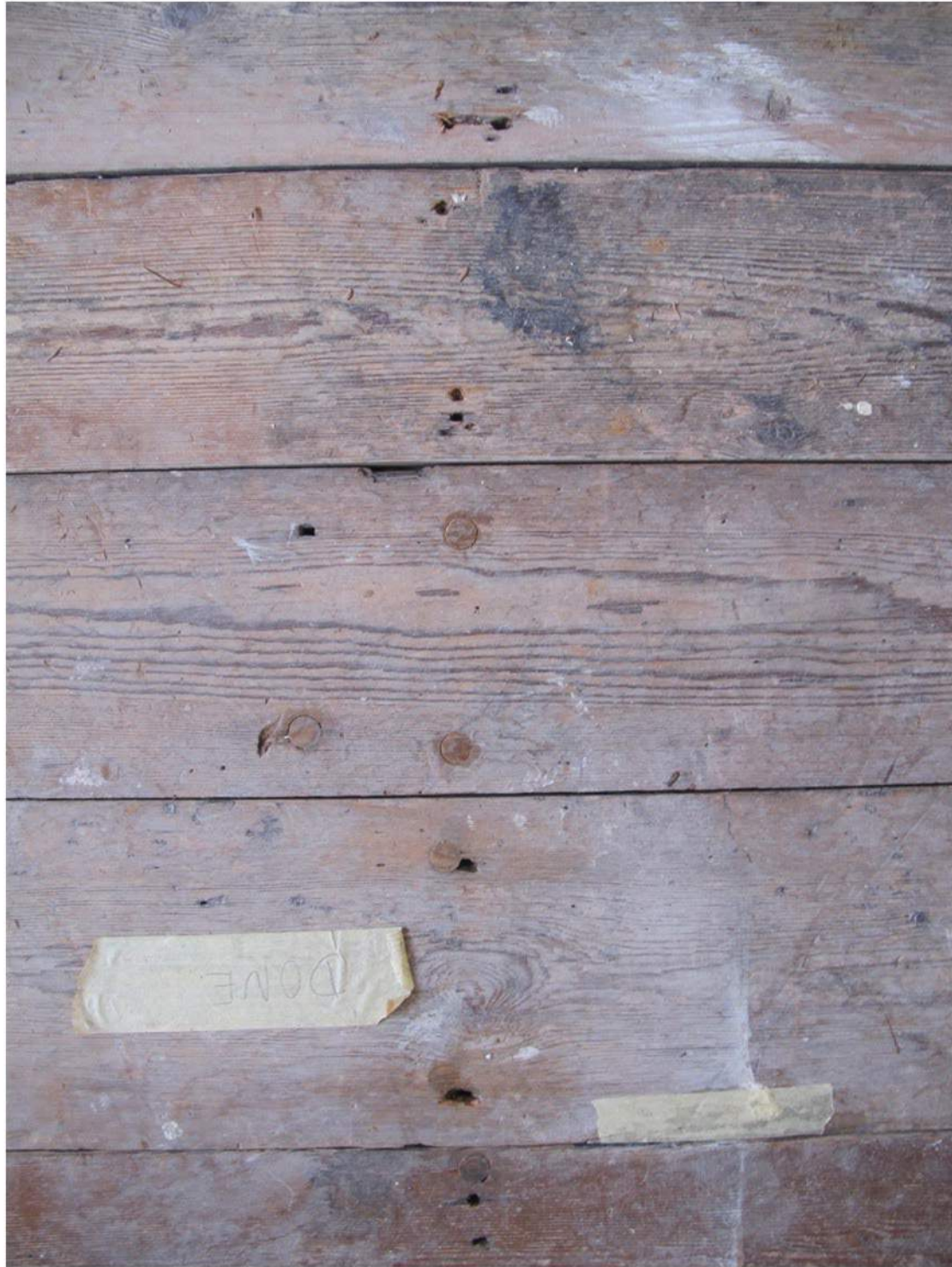
EXAMPLES OF PALETED FLOOR REPAIRS WHERE BOARDS HAD BEEN SCREWED INTO POSITION
