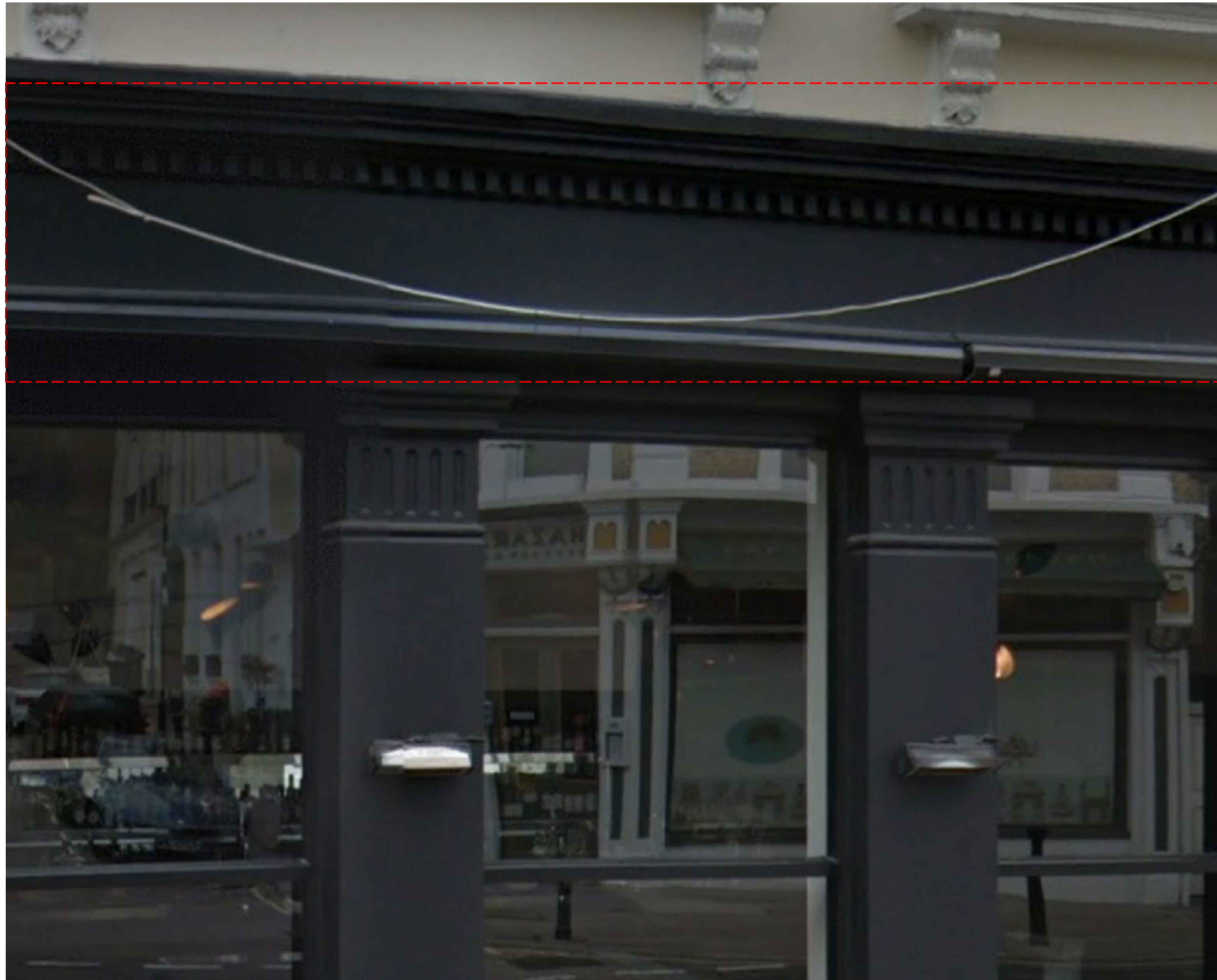
Cable to be tidied up
