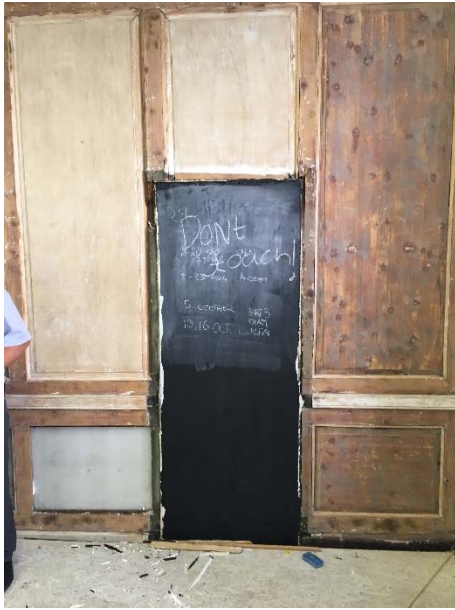
Fig 11 Non-original blackboard panel in RM.0.2
