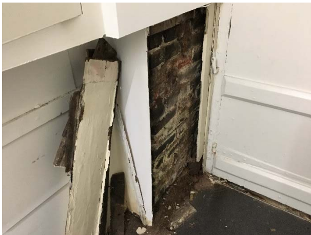
Fig 6 Damp seen in exterior brickwork
