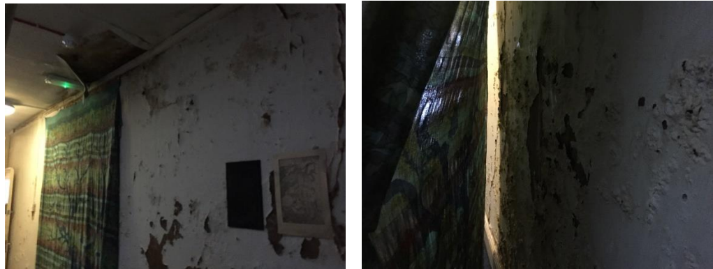
Figures 2 and 3: Water damage to interior wall of the hallway at the second floor level (Source: Icen Projects Ltd, Site visit conducted on 8 March 2017)
