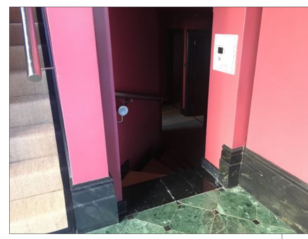
stair opening increased in width with dividing wall removed, stairs removed, skirtings and architraves removed
