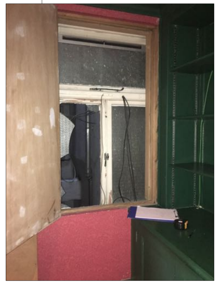
windows to be repaired and overhauled
