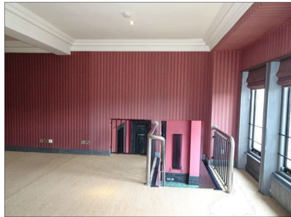
stair reconstructed within increased opening width and height. stairwell formed to flight serving lower floor level. flooring finishes, cornice and skirtings removed
