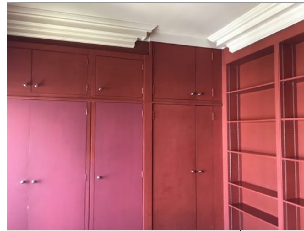
built in joinery closets and service cupds together with room cornice is to be removed
