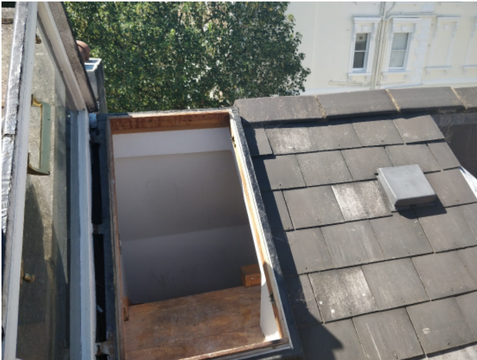
4) Narrow existing roof access
