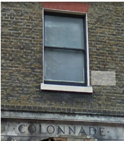
Figure 2: Horns on a window on the building's front elevation (Source: Google Streetview)
