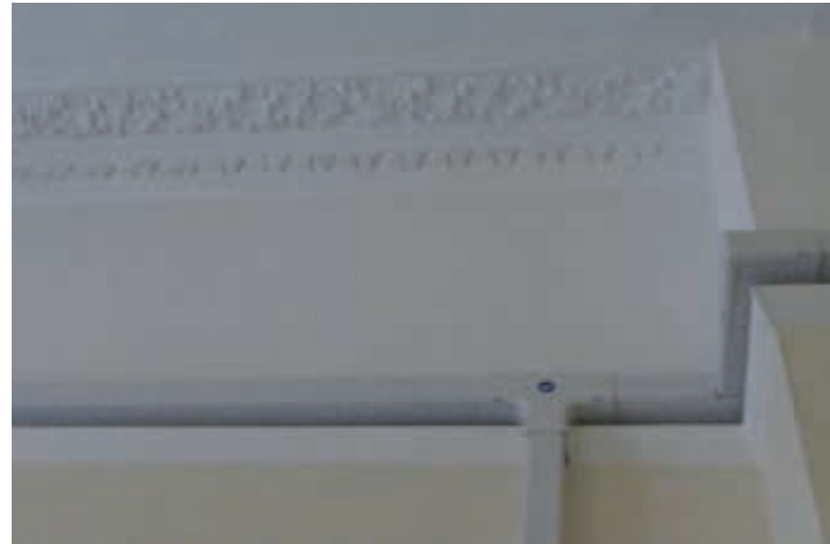
Figure 6.18 Boxed in services below cornice in no. 43
