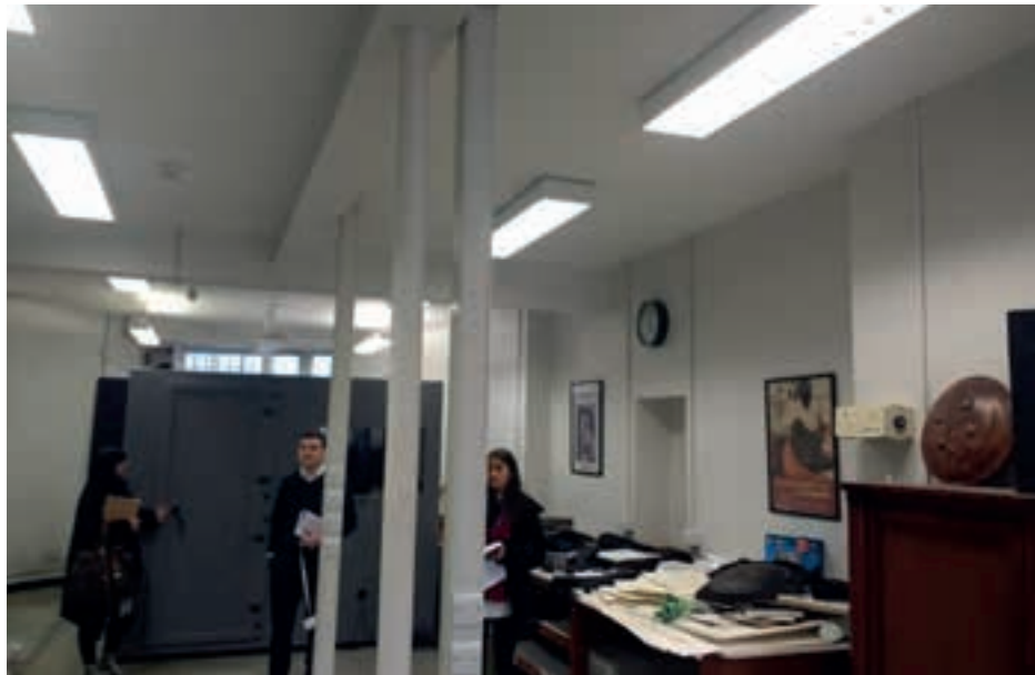
Figure 6.9 Vertical risers providing power in the middle of the basement space at no. 43
