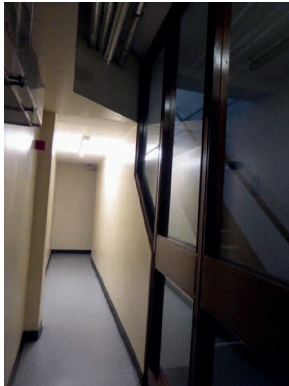
Figure 6.10 Glass partition at basement in no. 42- believed to have been introduced for fire safety to separate off the staircase as part of office conversion works
