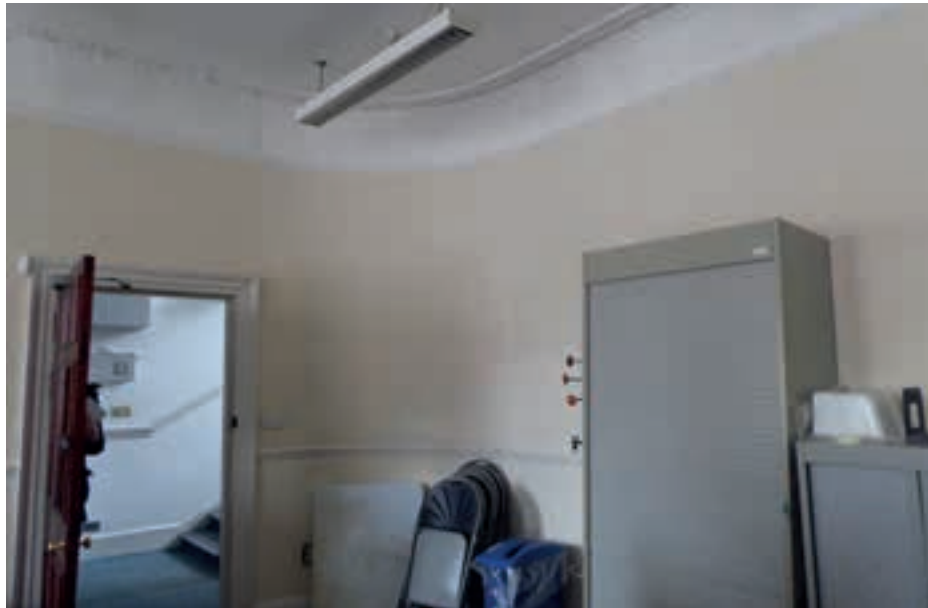
Figure 6.14 Ground floor main room at 43 showing original curved wall between principal rooms
