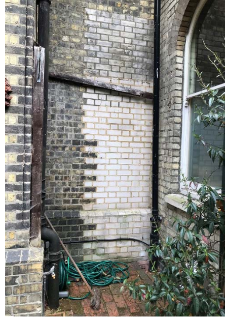
10.5 Bay and RH wall behind with blocked door
