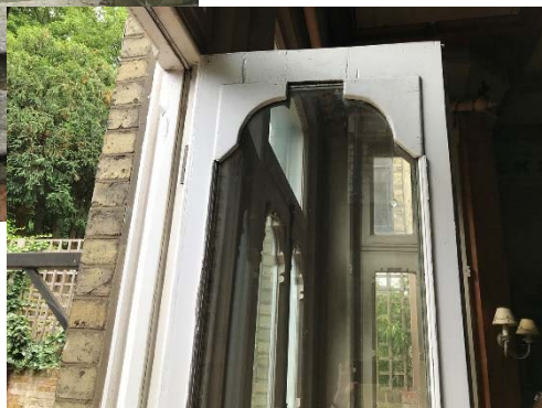
12.2 Poor detailing and applied plywood mouldings
