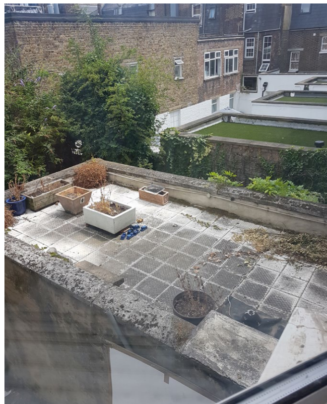
View of rear extension to No. 200 (looking out of upper floor window from No. 202)
