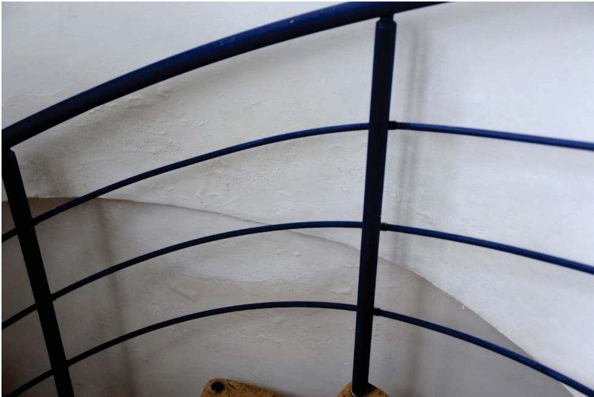
Fig 38 The wall affected by damp at ground floor level in the north-west tower
