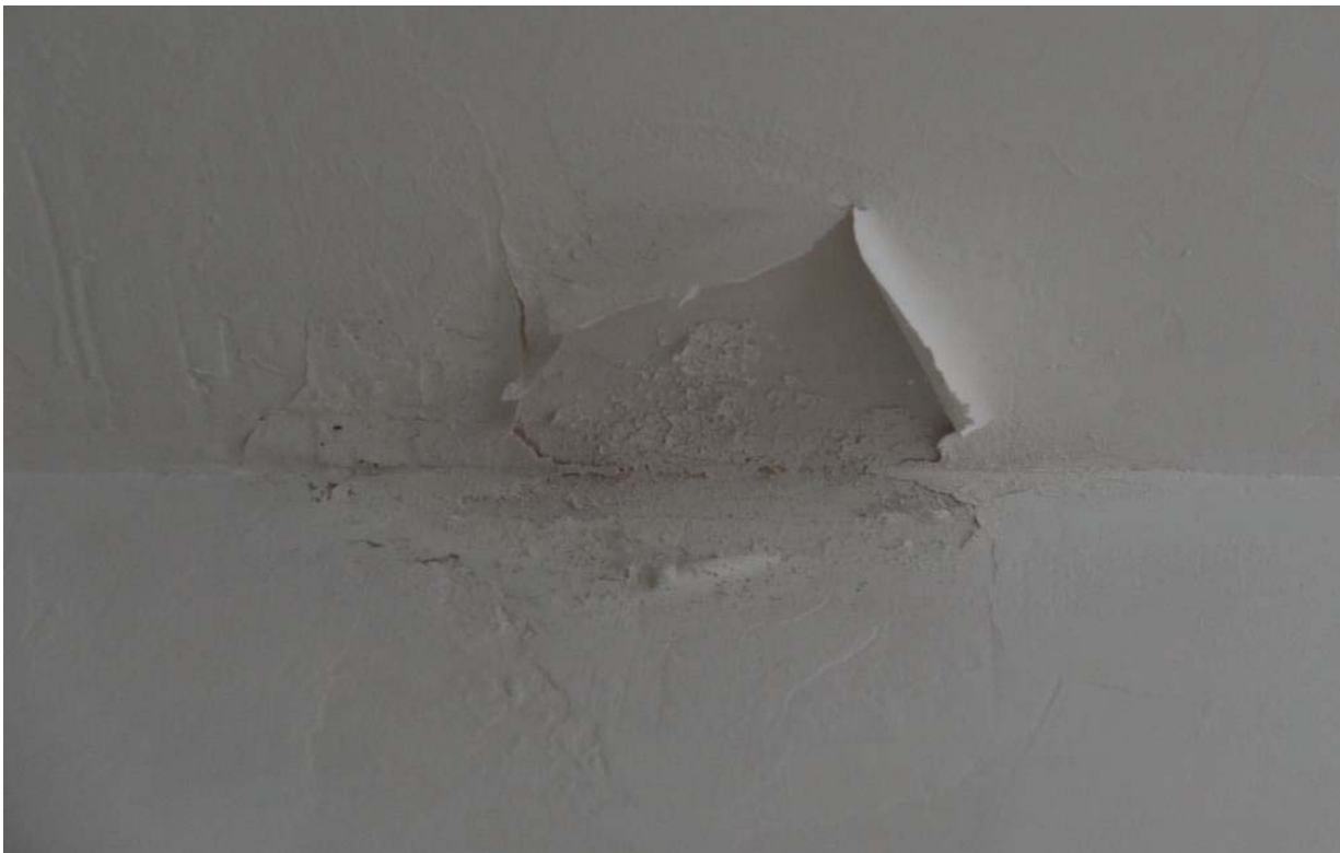
Fig 24 The damp ingress on the ceiling and south wall of the passage in the basement
