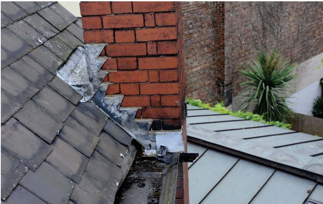
Fig 9 The cast iron gutter and lead flashings at the base of the east chimney stack
