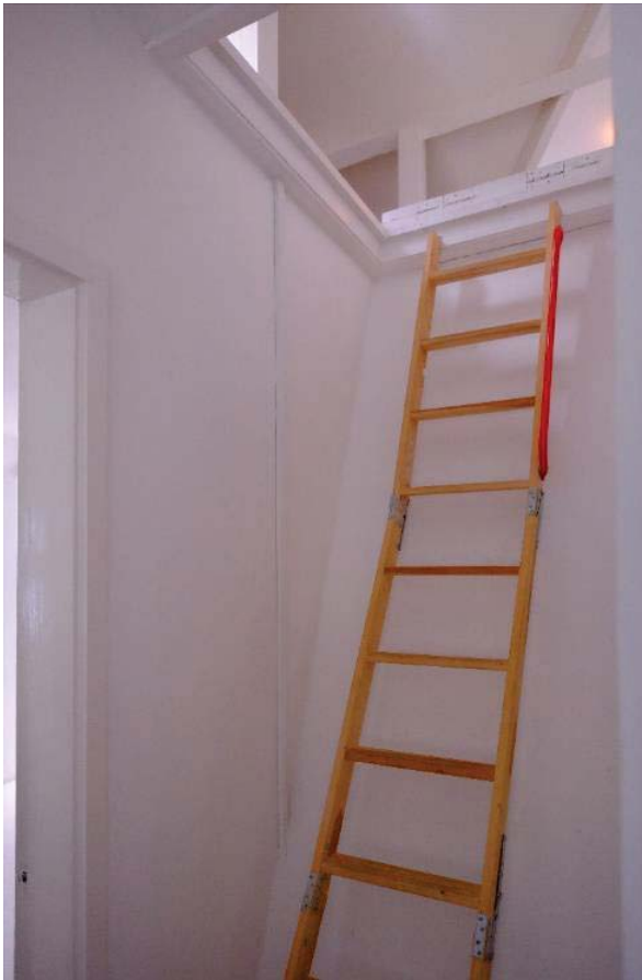
Fig 46 The loft ladder and attic access hatch
