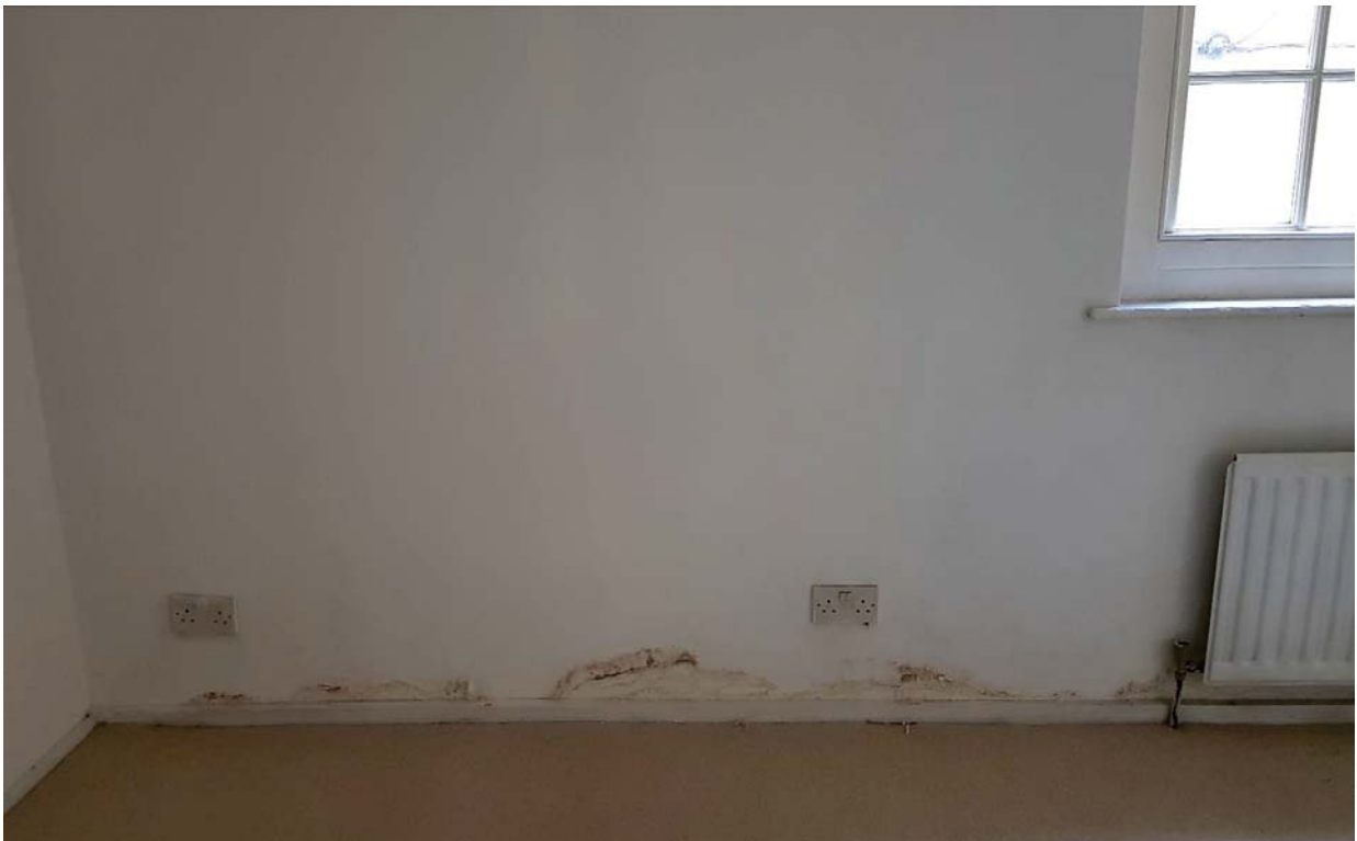
Fig 55 The damp on the west wall
