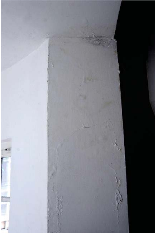
Fig 30 The damp ingress on the wall at the transition between the north-west tower and north room on the first floor
