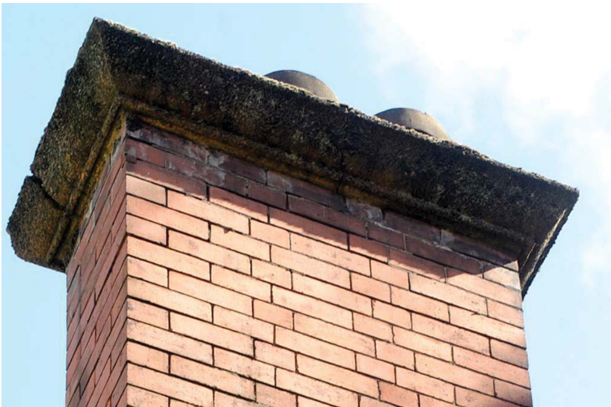
Fig 11 The cracked concrete cap of the south chimney stack
