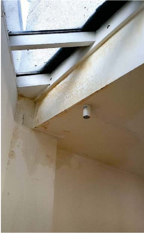
Fig 53 The damp at the south end of the glazed roof on the ground floor.
