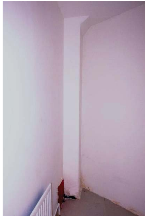
Fig 42 The damp ingress at the bottom of the north-east pier in the south-east room of the basement
