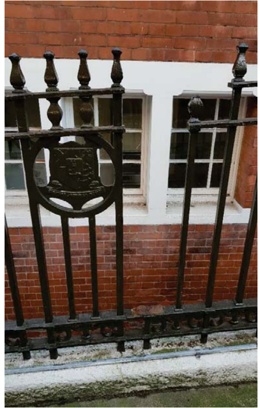
Fig 54 The damaged railing on the north boundary.
