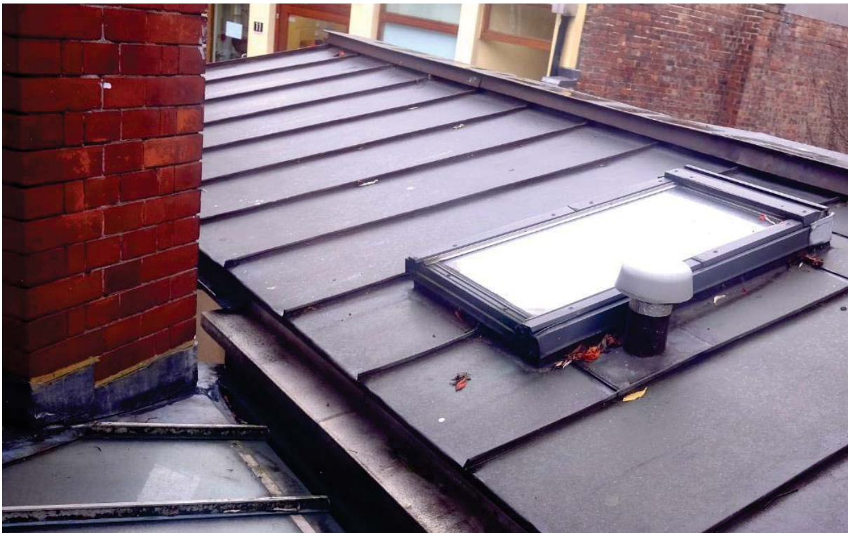
Fig 37 The gutter detail between the east wall of The Lodge and the adjacent property
