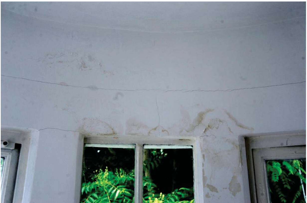
Fig 29 Damp staining above window W50
