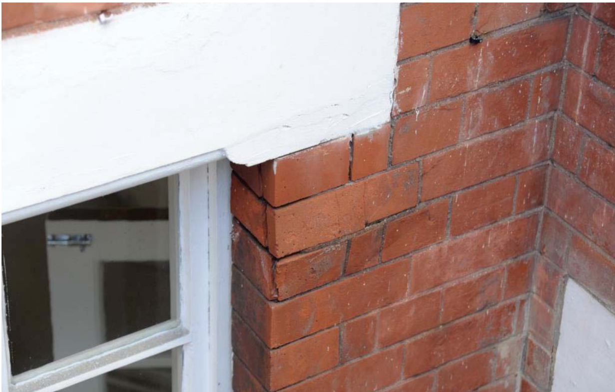
Fig 16 An earlier repair to the south jamb of window W27
