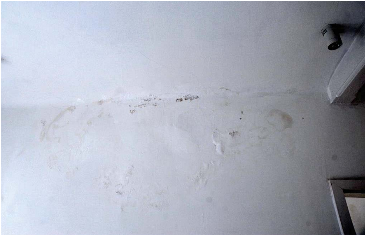
Fig 28 The damp ingress on the south wall of the stair
