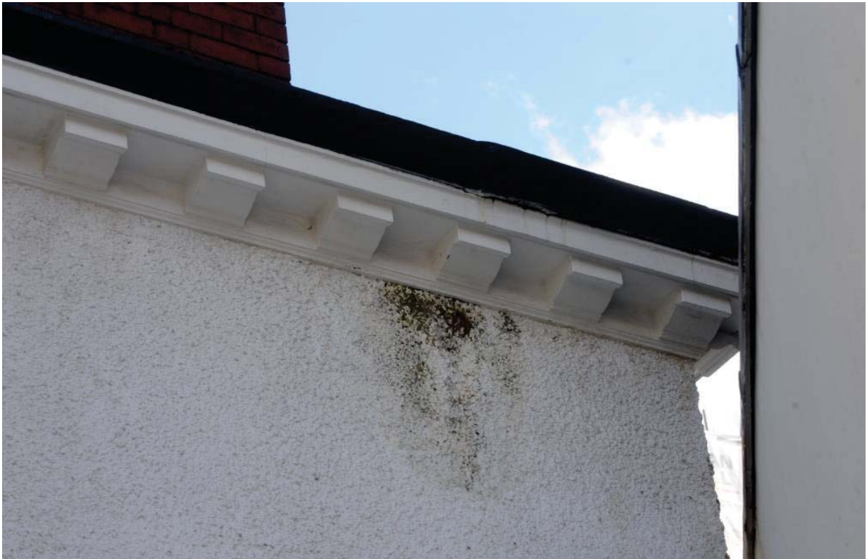
Fig 10 Algae staining of the render under a defective gutter on the south elevation
