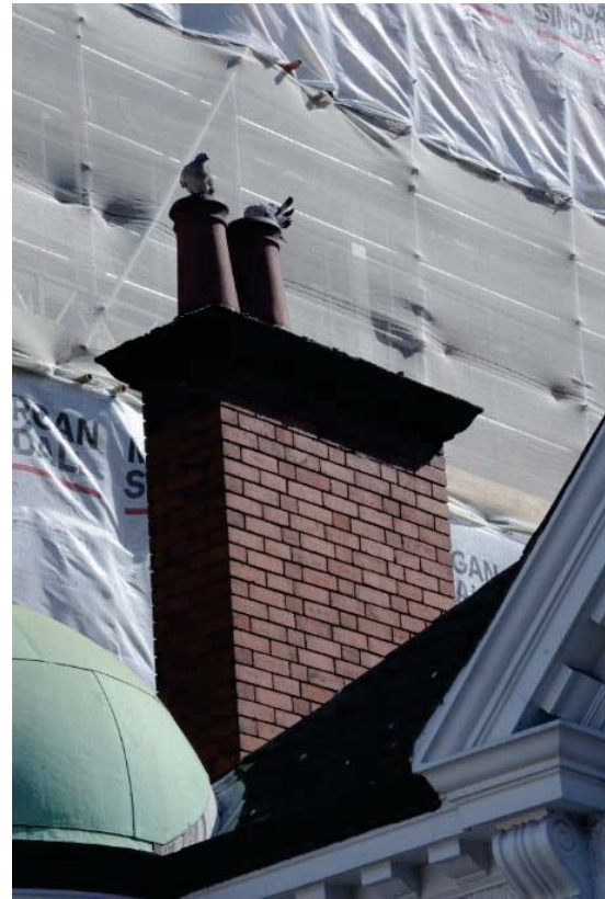
Fig 13 The north chimney stack
