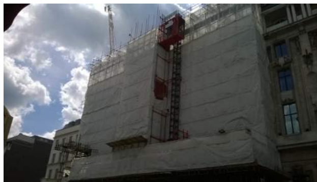
Figure 12: The site setup at High Holborn will be similar to our setup at 50 St James's Street, with sheeted access scaffolds, a lifting beam and a goods hoist.
