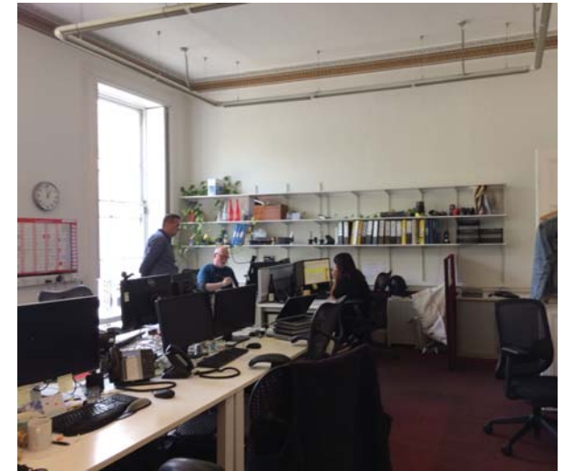
Surface mounted lighting in front office.
