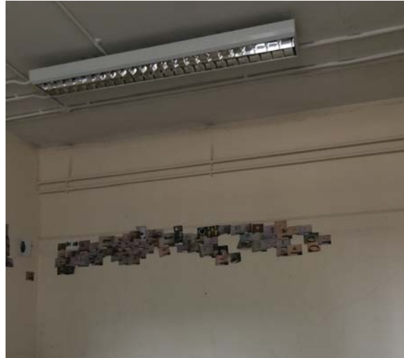
Front room surface mounted conduits.
