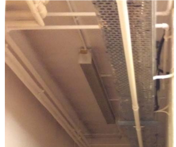
Exposed cables trays and services pipes.
