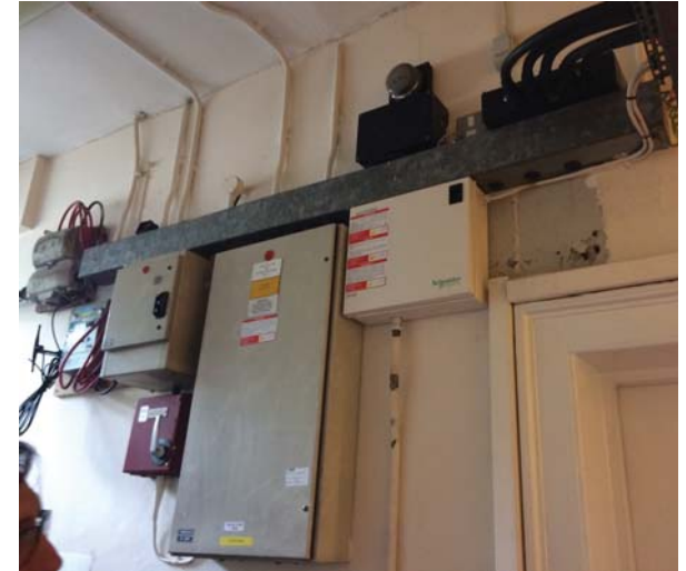
Exposed services at high level.
