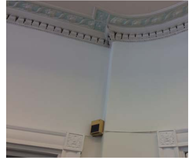
Surface mounted conduits and cables in front office above door architraves.
