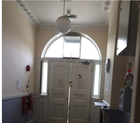
Surface mounted conduits and cables in entrance lobby.
