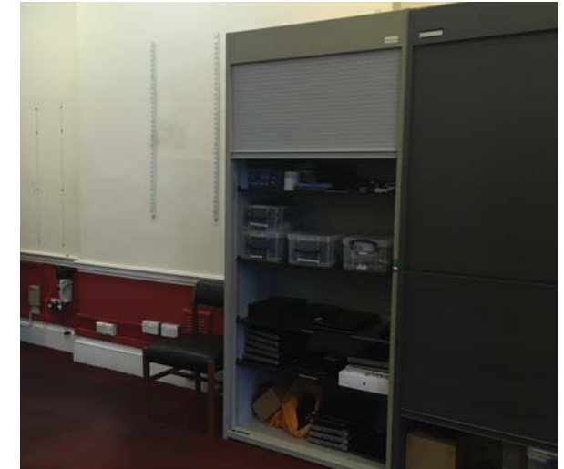
Surface mounted services below dado rail.
