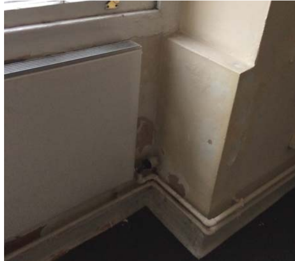
Damp below front room window.
