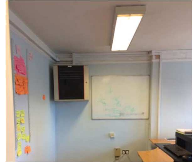
Front office with surface mounted services.
