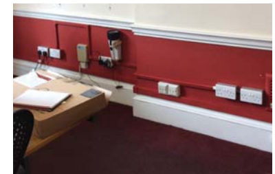
Above: 41 Russell Square - The images above show the approach towards the surface mounted services adopted throughout.
