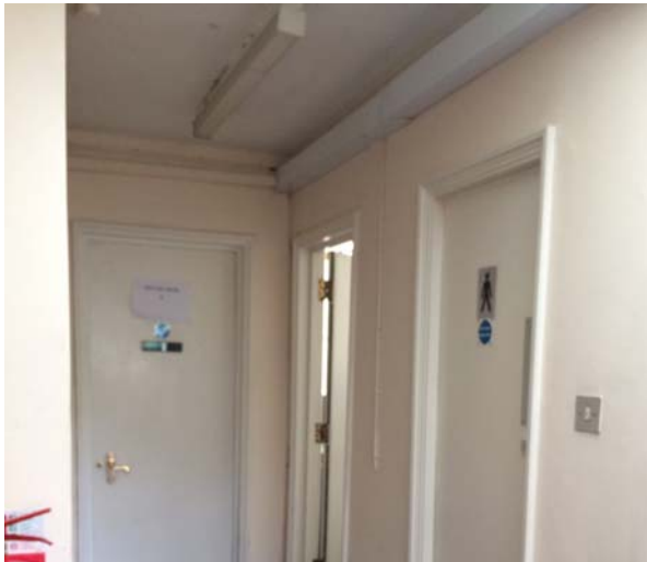
Corridor and ducts at high level.
