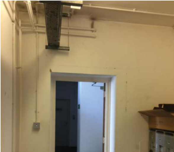
Services ducts and missing architrave.
