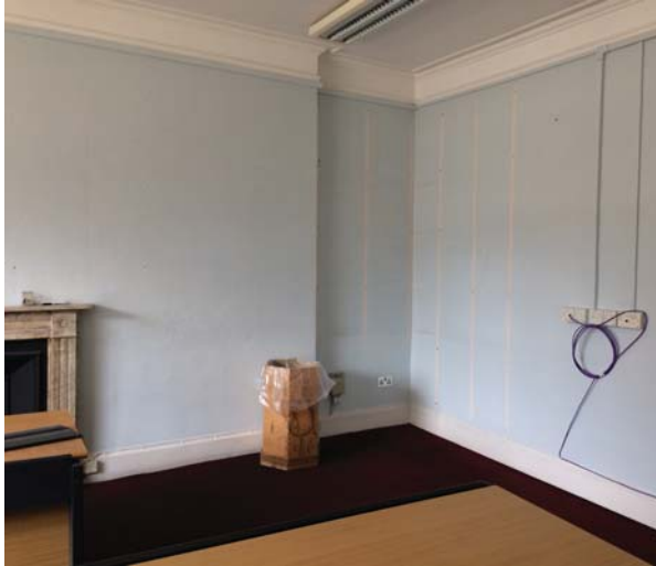
Looking at existing blocked up fireplace and exposed services in rear office
