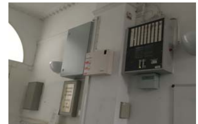
Above: 42-43 Russell Square - The images above show the approach towards the surface mounted services adopted throughout.
