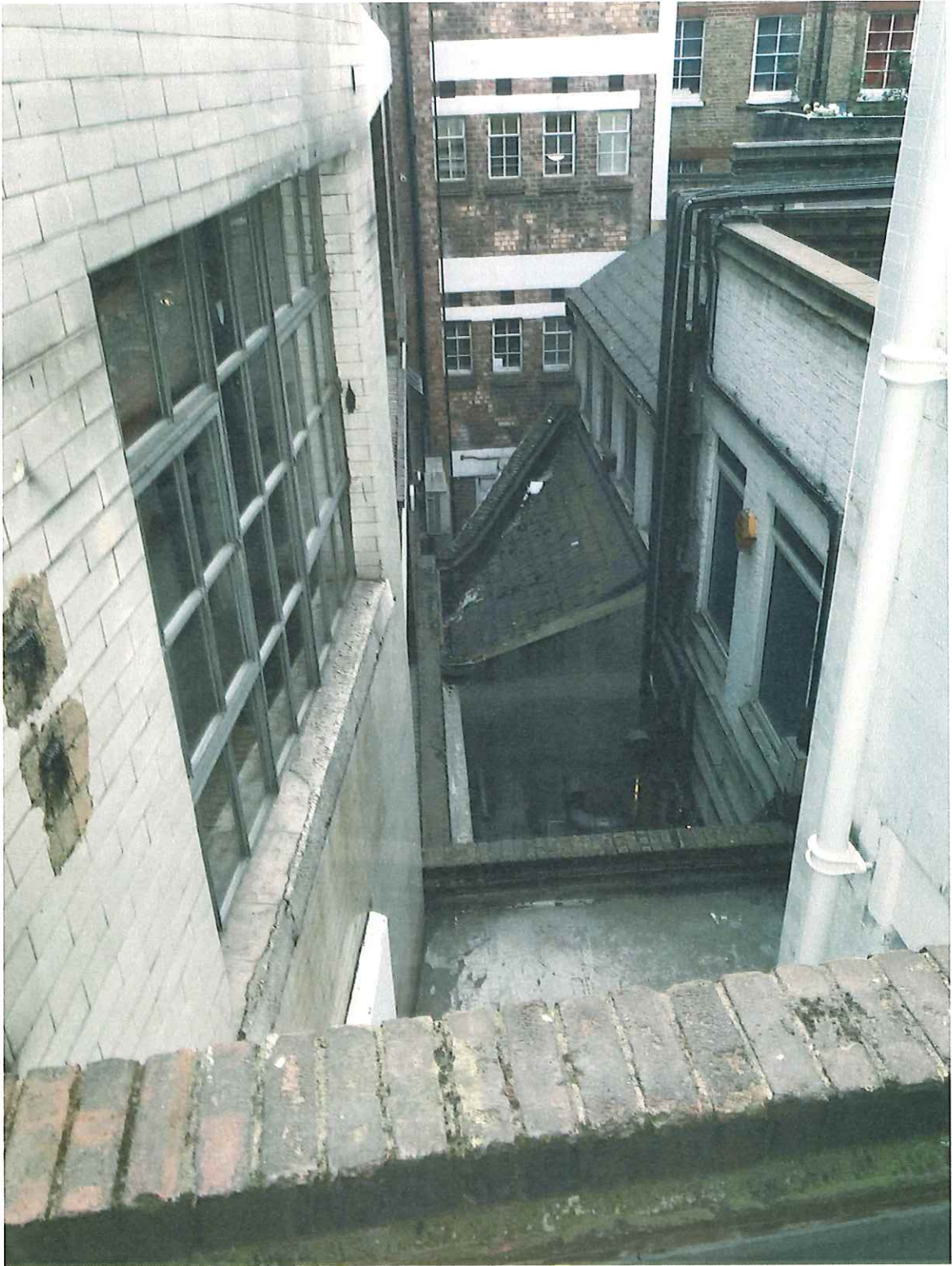
Photo N – Ground Floor HRU intake & discharge in basement light well
