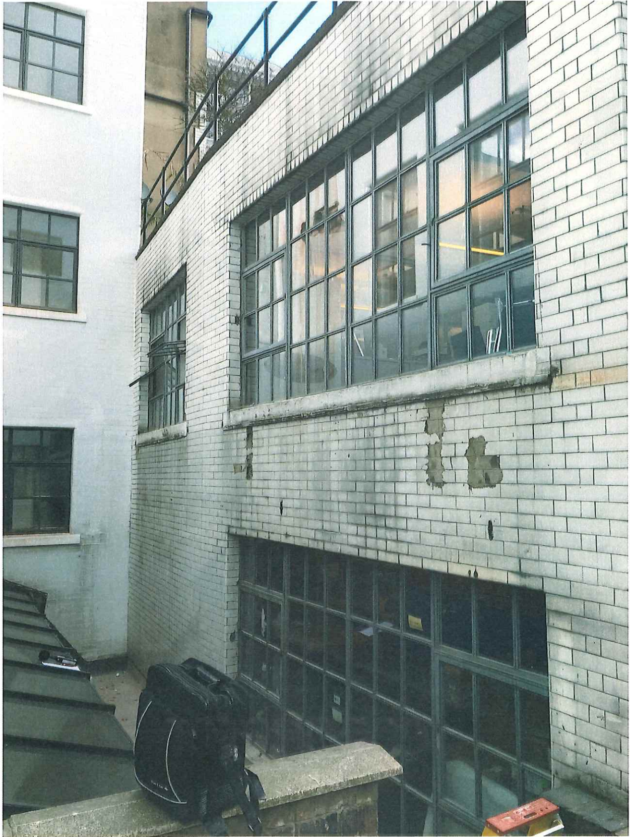
Photo M – Office windows immediately opposite 1 st , 2 nd & 3 rd floor HRU intakes/discharges
