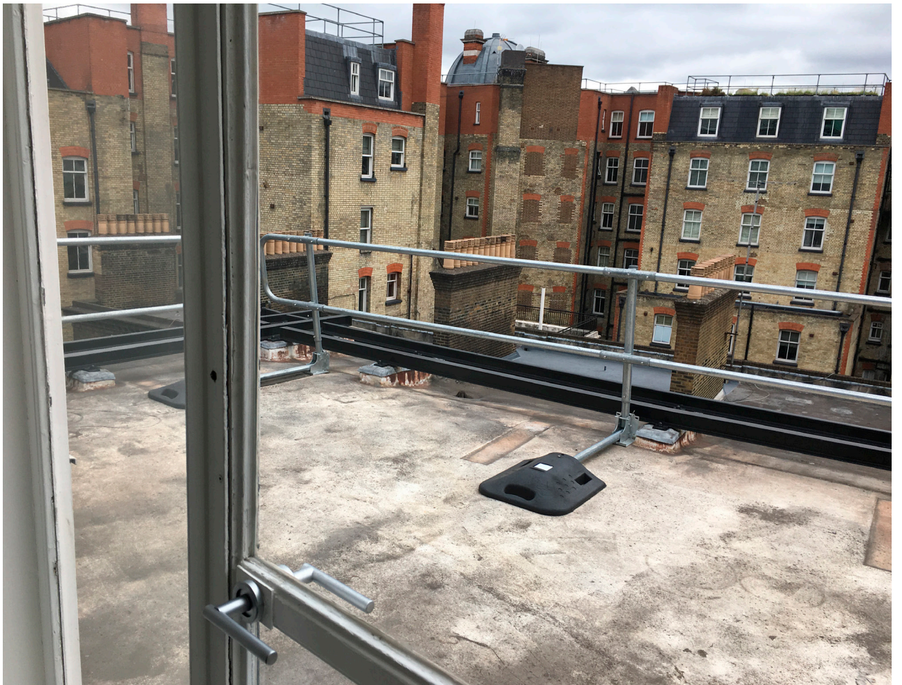
Views of the existing roof area looking south-east (above) and north-east (below)
