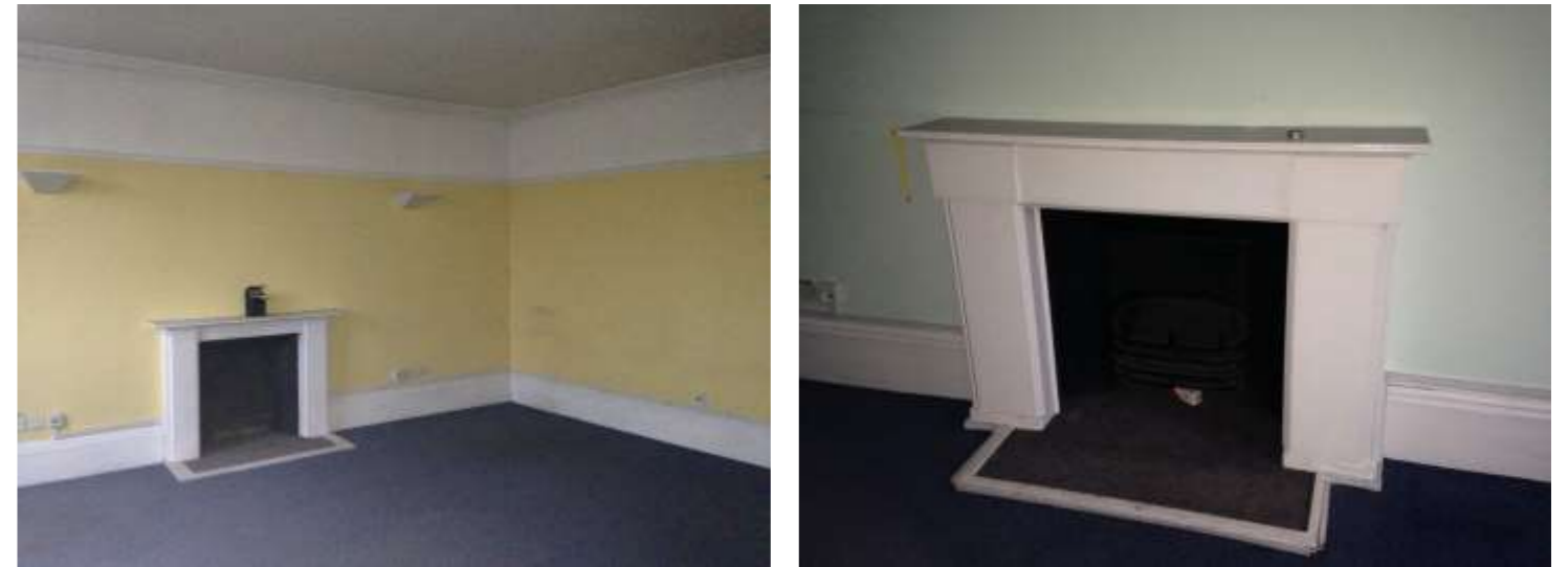
Figure 15: Office to the second floor, showing fireplace and surrounds with skirting, picture rails and cornicing.
