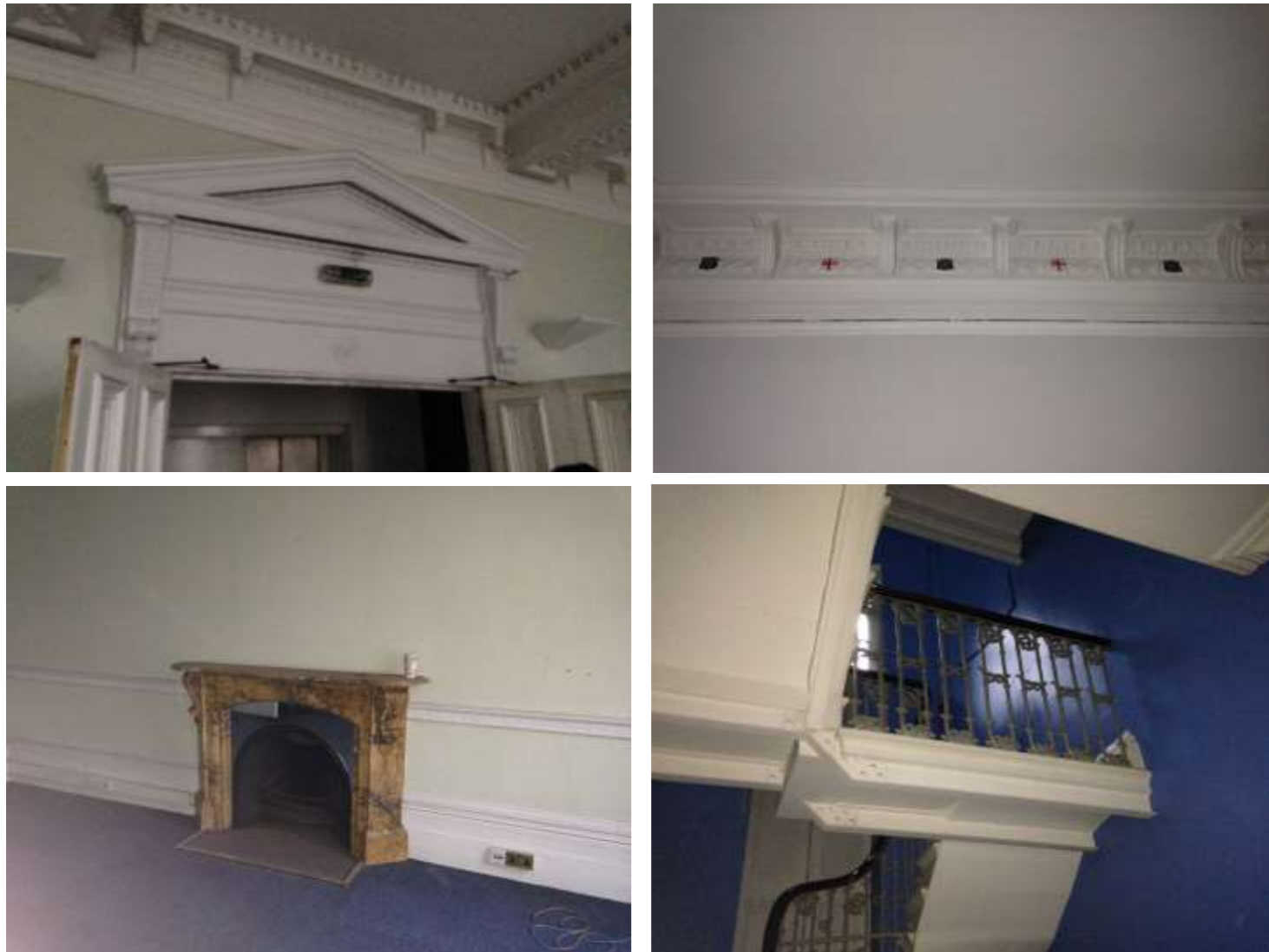
Figure 14: Pediment joinery over door between front and rear office on the first floor (top left), decorative cornicing with painted emblems and crests on first floor (top right), fireplace surround to first floor (bottom left) and cantilevered landing to staircase between first and second floors (bottom right).
