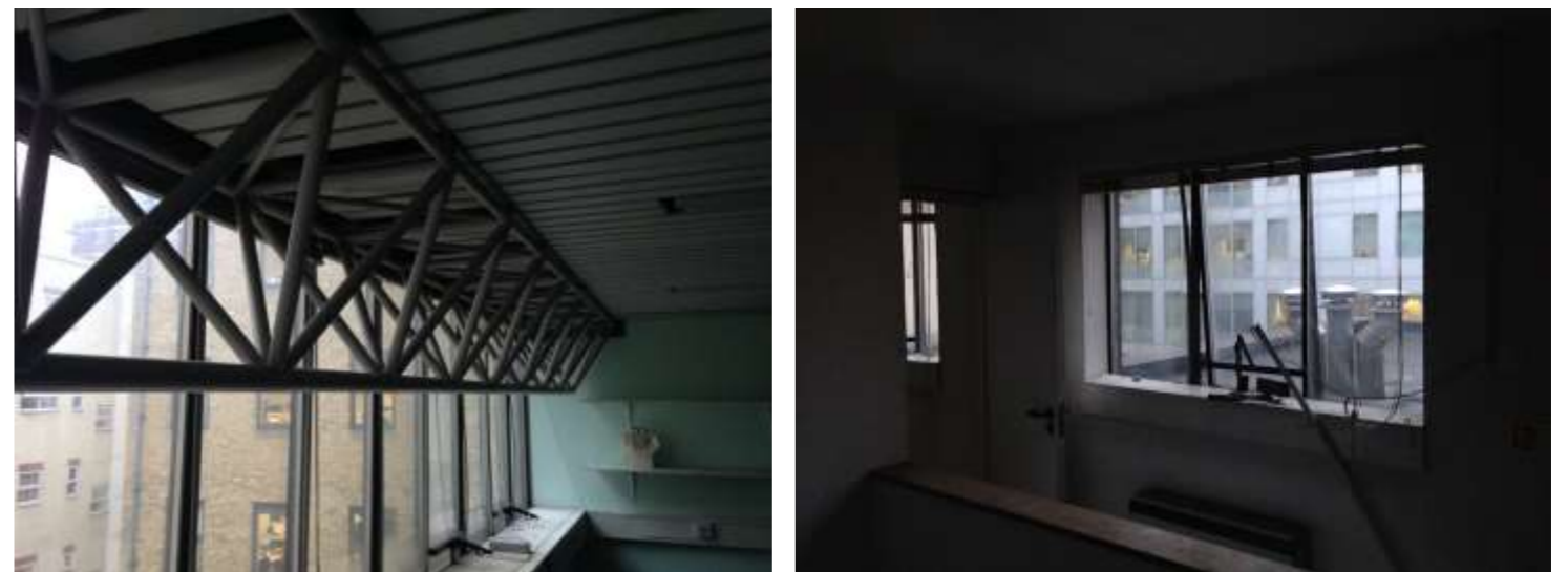
Figure 16: Large rear office to the third floor with modern structural element (left) and landing area to the fourth floor (right).
