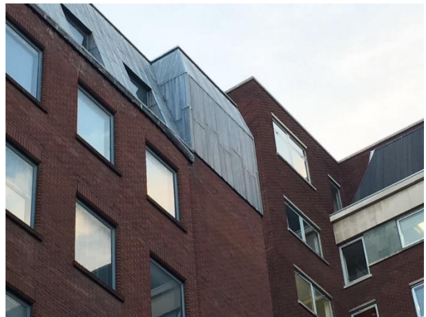
Photograph 4: Upper section of building as viewed from the central courtyard of 150 Holborn
