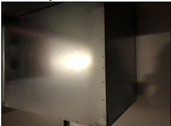
Photo.1.5. Atmospheric side attenuator installed on Extract fan - See Drawing L1975M004
