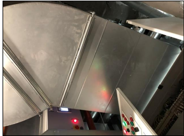
Photo.1.2 Atmospheric side attenuator installed on AHU 2 See Drawing L1975M003
