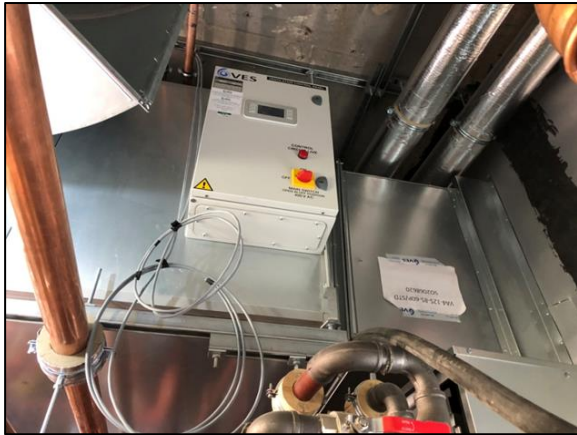
Photo.1.1. Atmospheric side attenuator installed on AHU 1 See Drawing L1975M003
