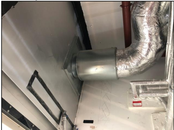
Photo.1.3. Atmospheric side attenuator installed on AHU 3 See Drawing L1975M003
