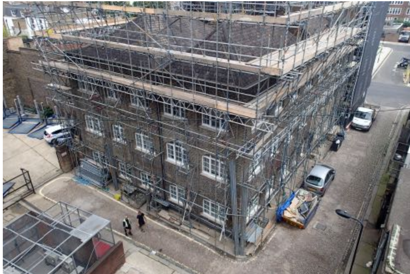
3 storey addition underway to 48-56 Bayham Place utilising brick lacework and zinc cladding to the upper storeys.
