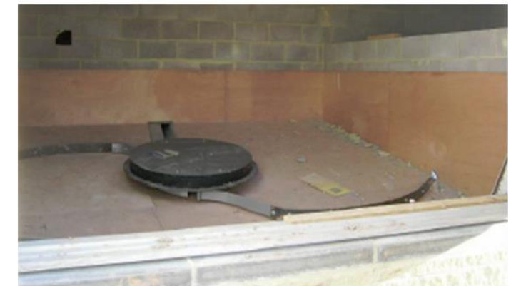
Typical Wood Pellet Feeder
