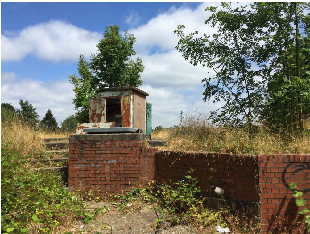
Plate 2: Utilitarian above ground structures within the Site boundary associated with the former reservoir, including a number of vents.
