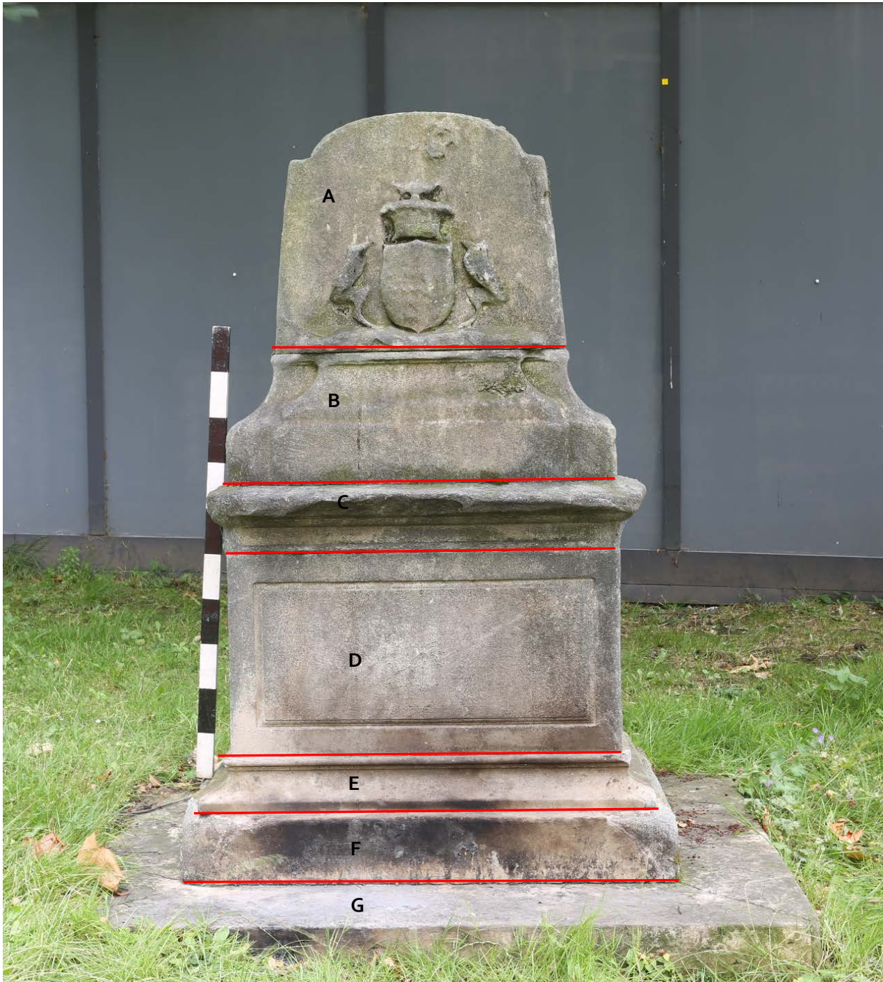
Figure 8 North Elevation of monument annotated to show bed joints and course labelling
