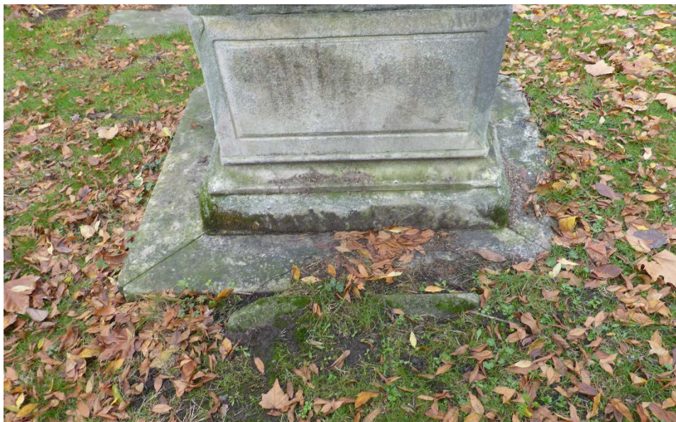
Figure 4 Partially buried section of stone on the south side of the obelisk
