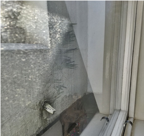
front gutter detail below cill level
