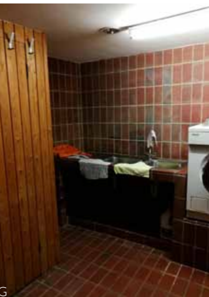
Photos D-G These photos show boxing in to the original lightwell windows as well as the remains of an original arch to the kitchen hearth which now holds new boiler. Photo G shows utility area to the back of the basement.
