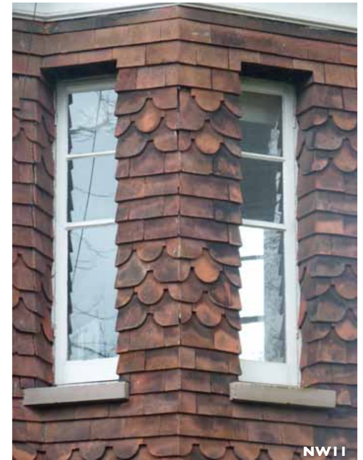
Photos NW9-NW11 Existing first floor windows on North -West Elevation. The sash windows seem to be original. The casement windows in the corner bay seem to be original as well.
