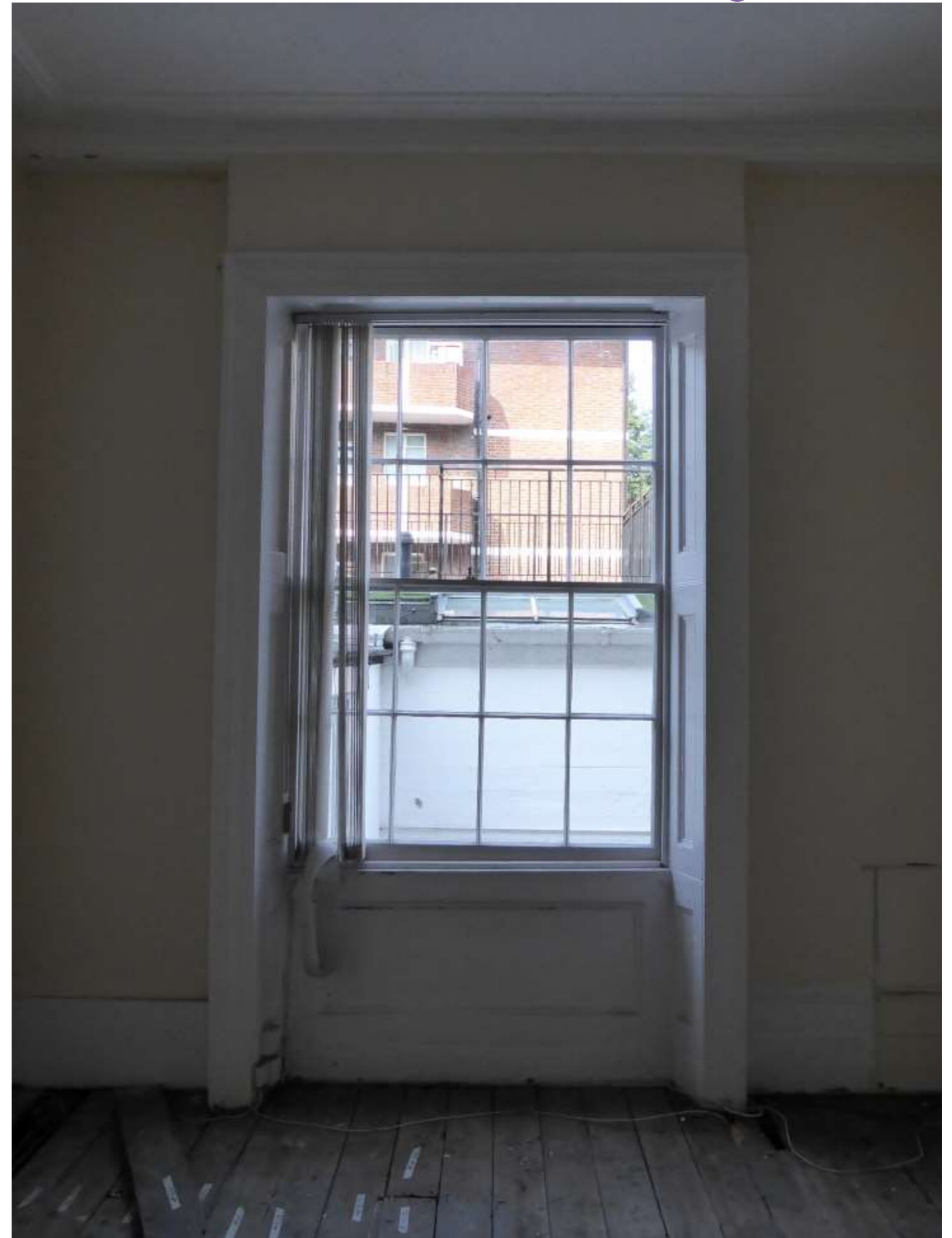
Plate F1: The first floor rear window with shutterbox standing proud of with the walls either side.
