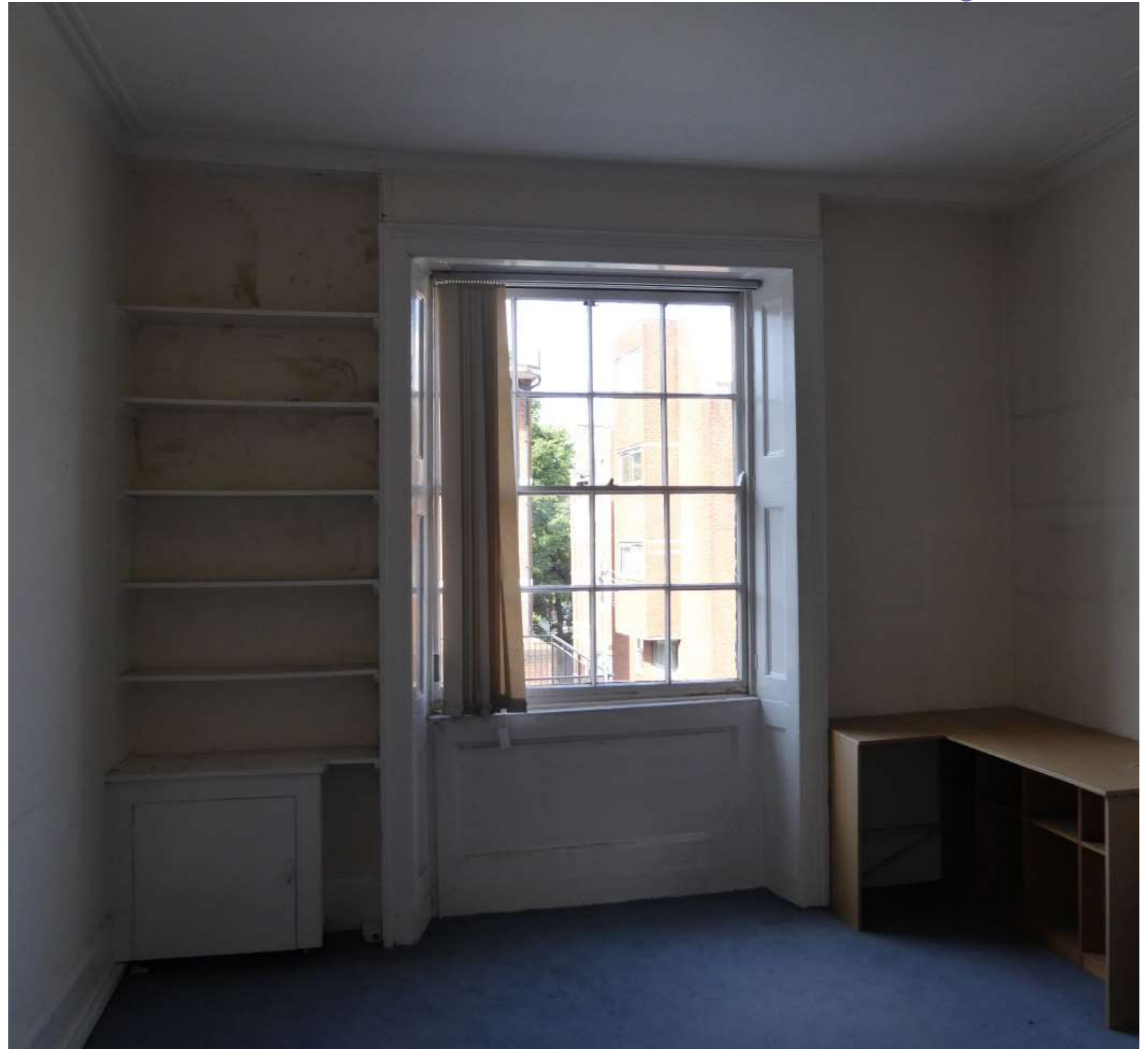
Plate S1: The second floor rear window with shutterbox standing proud of with the walls either side.
