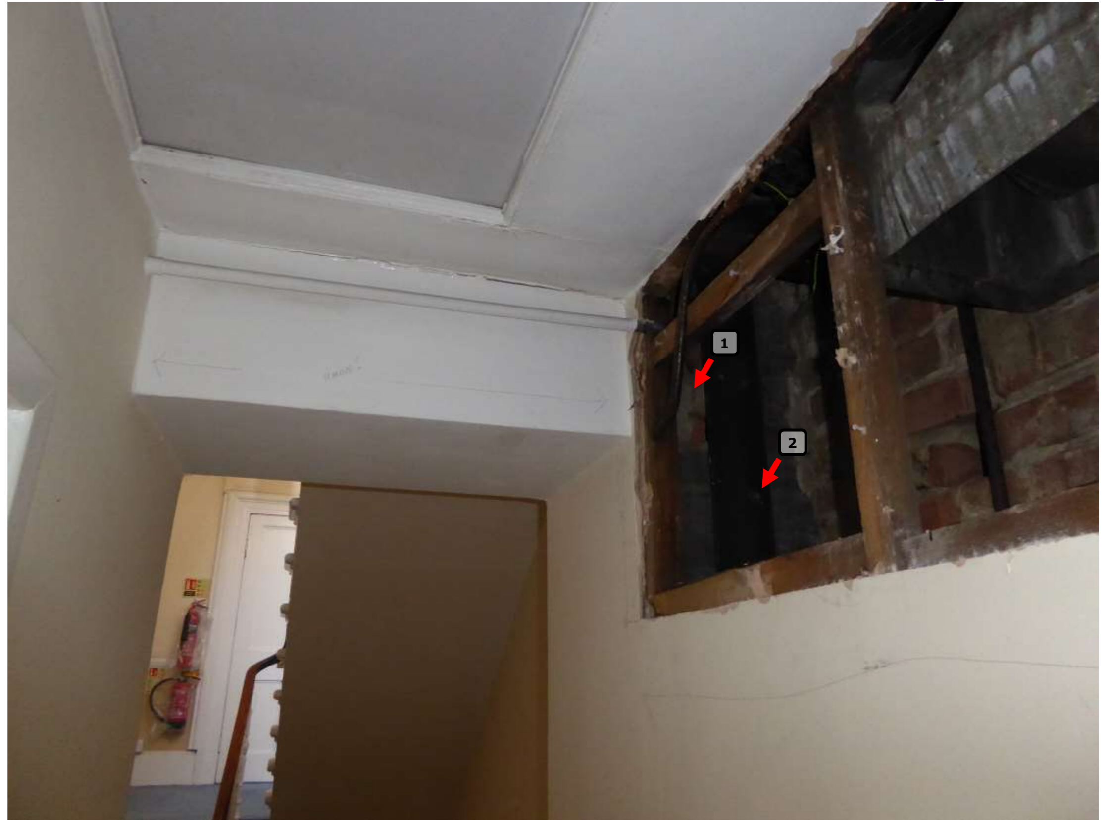
Plate FL1: The area that has been opened up. Note the down pipe [2] and the concrete lintol spanning the opening [1]. The down pipe can be seen externally at Plate E2 on page 15.
