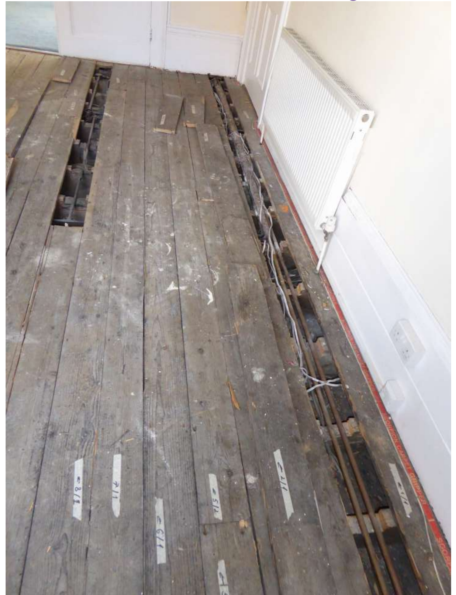
Plate F2: The existing pipe runs in notches, from the rear looking towards the front.
