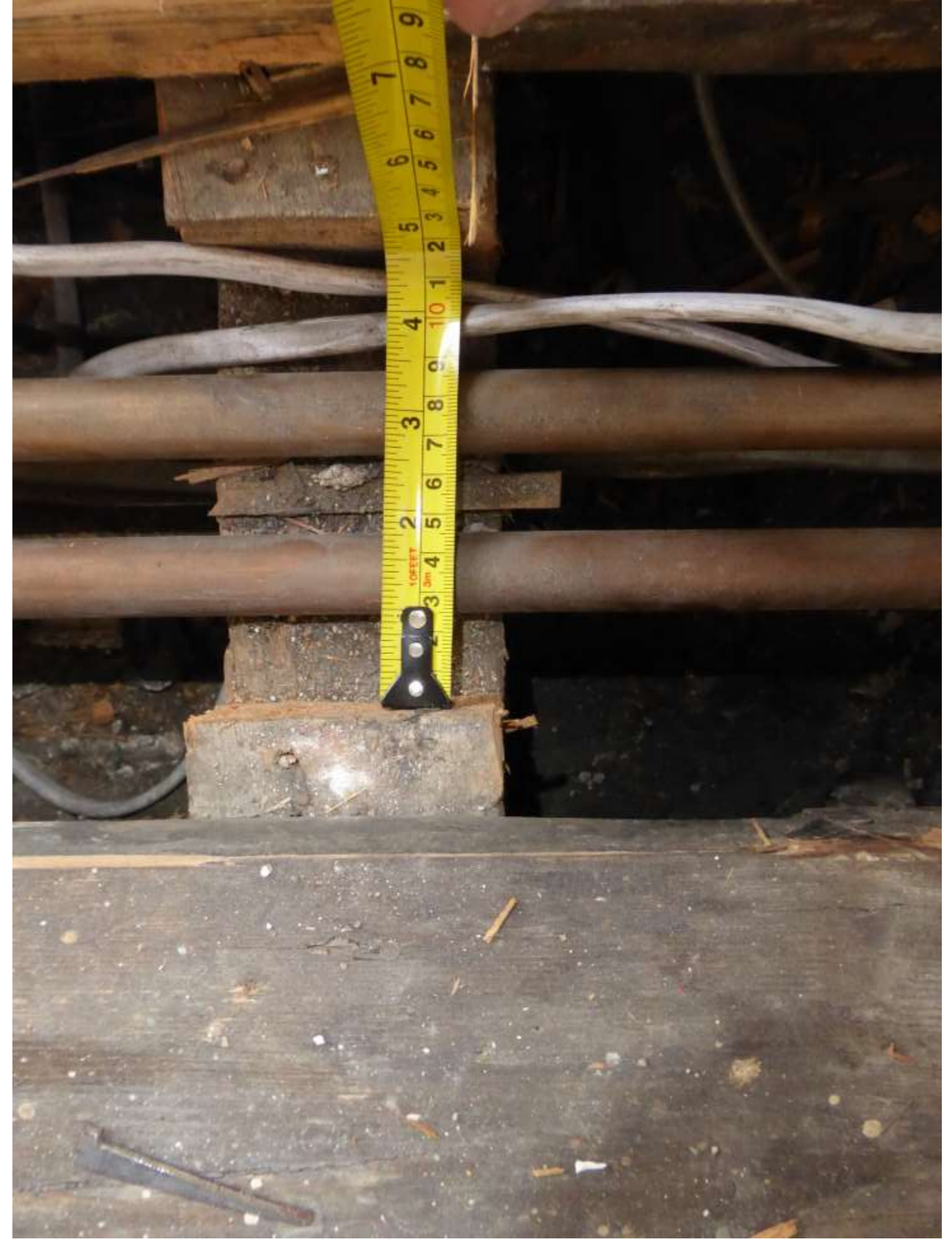
Plate F3: Detail showing the width of the existing pipe run closest to the stairs.
