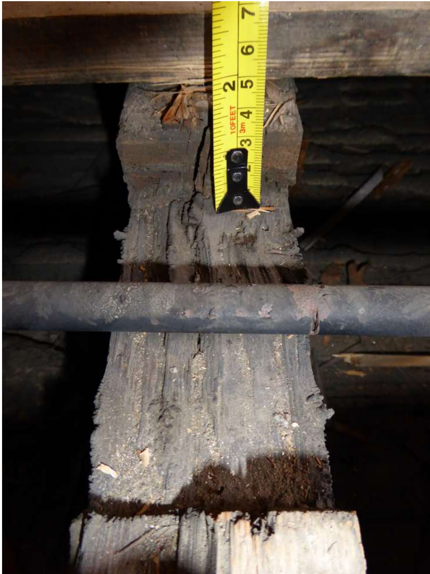
Plate F4: Detail showing the depth of the existing pipe run furthest from the stairs.
