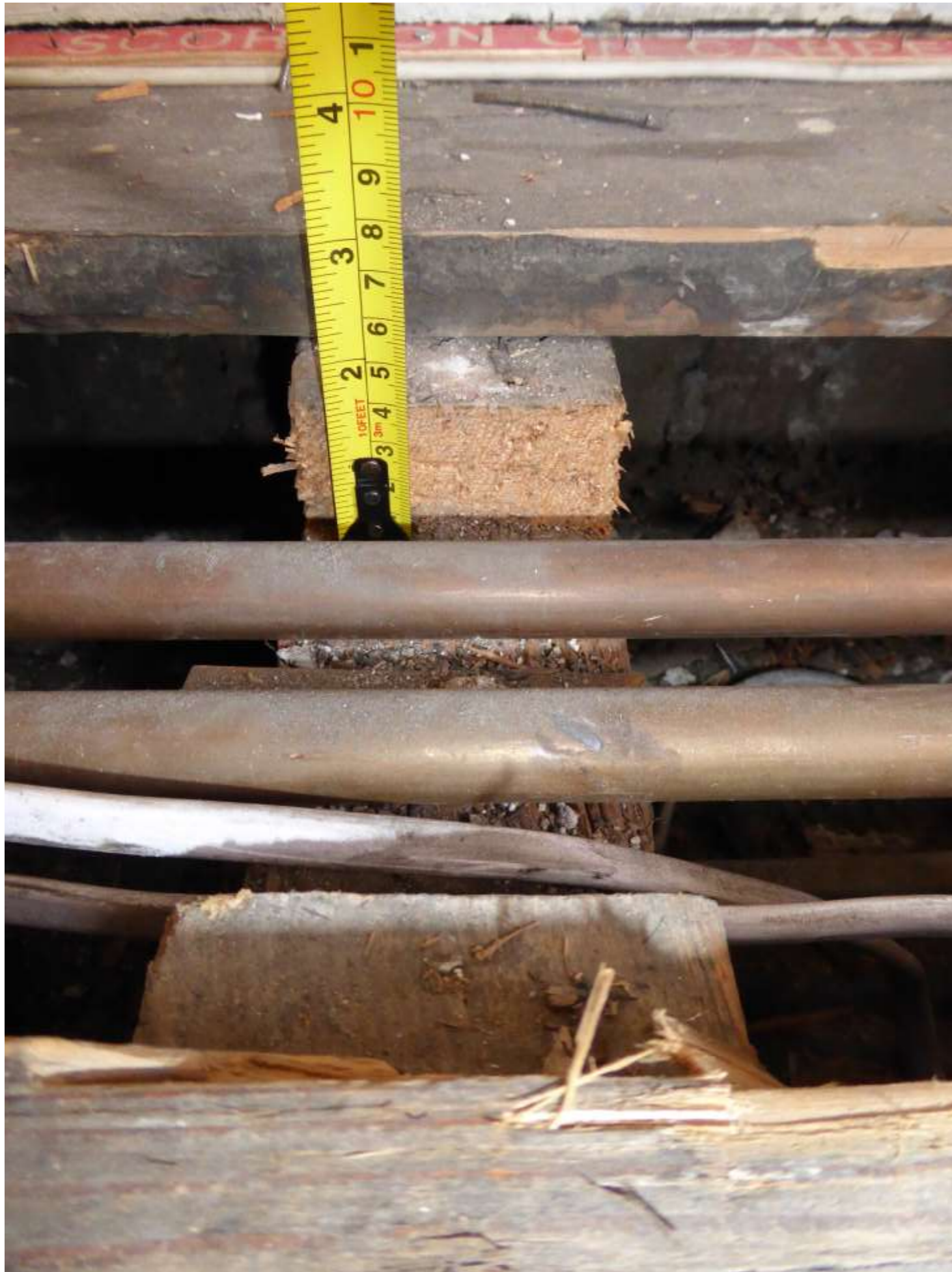
Plate F3: Detail showing the depth of the existing pipe run closest to the stairs.
