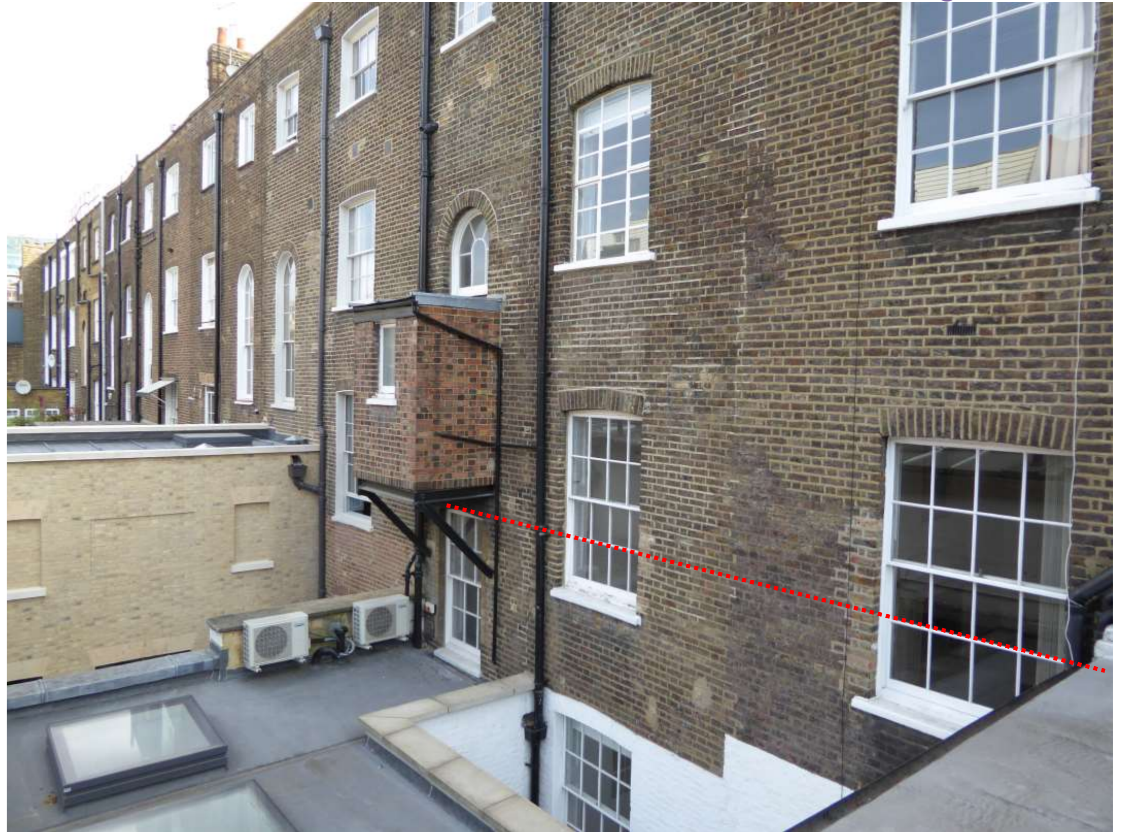
Plate E1: The rear elevation, showing an original first landing stairs window, underneath the arched second landing window. The red line shows the approximate height of the window head.
