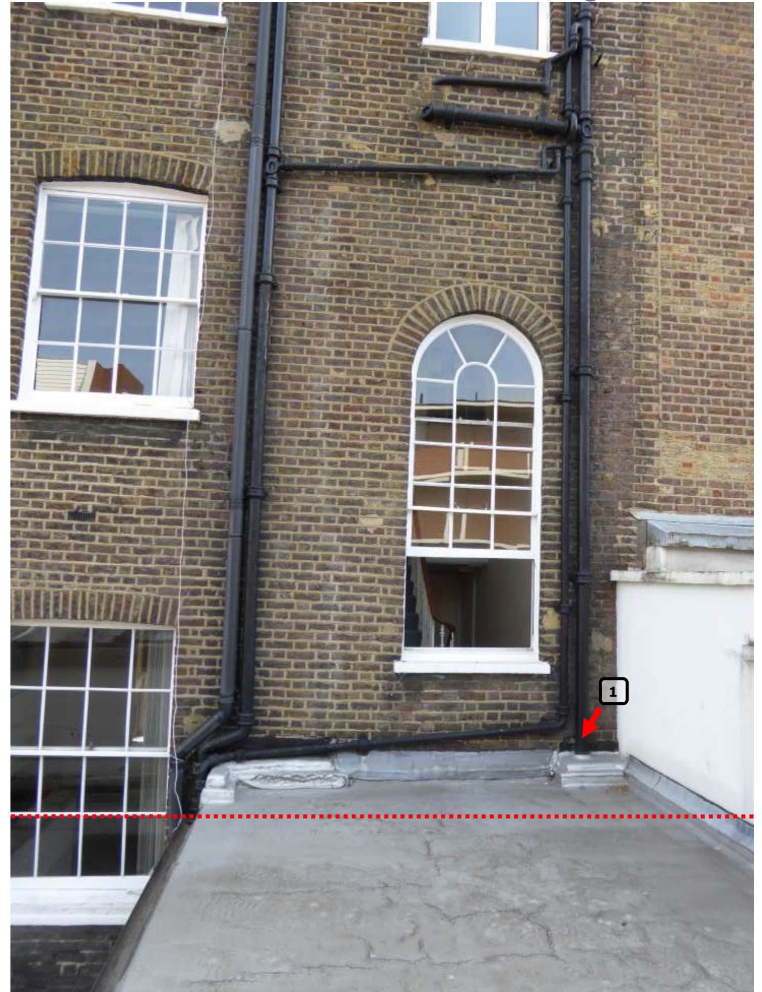
Plate E2: The rear elevation of No. 28 with the red line extrapolated from the previous photo. The down pipe [1] can be seen internally at Plates FL1 and FL2 on pages 12 & 13.
