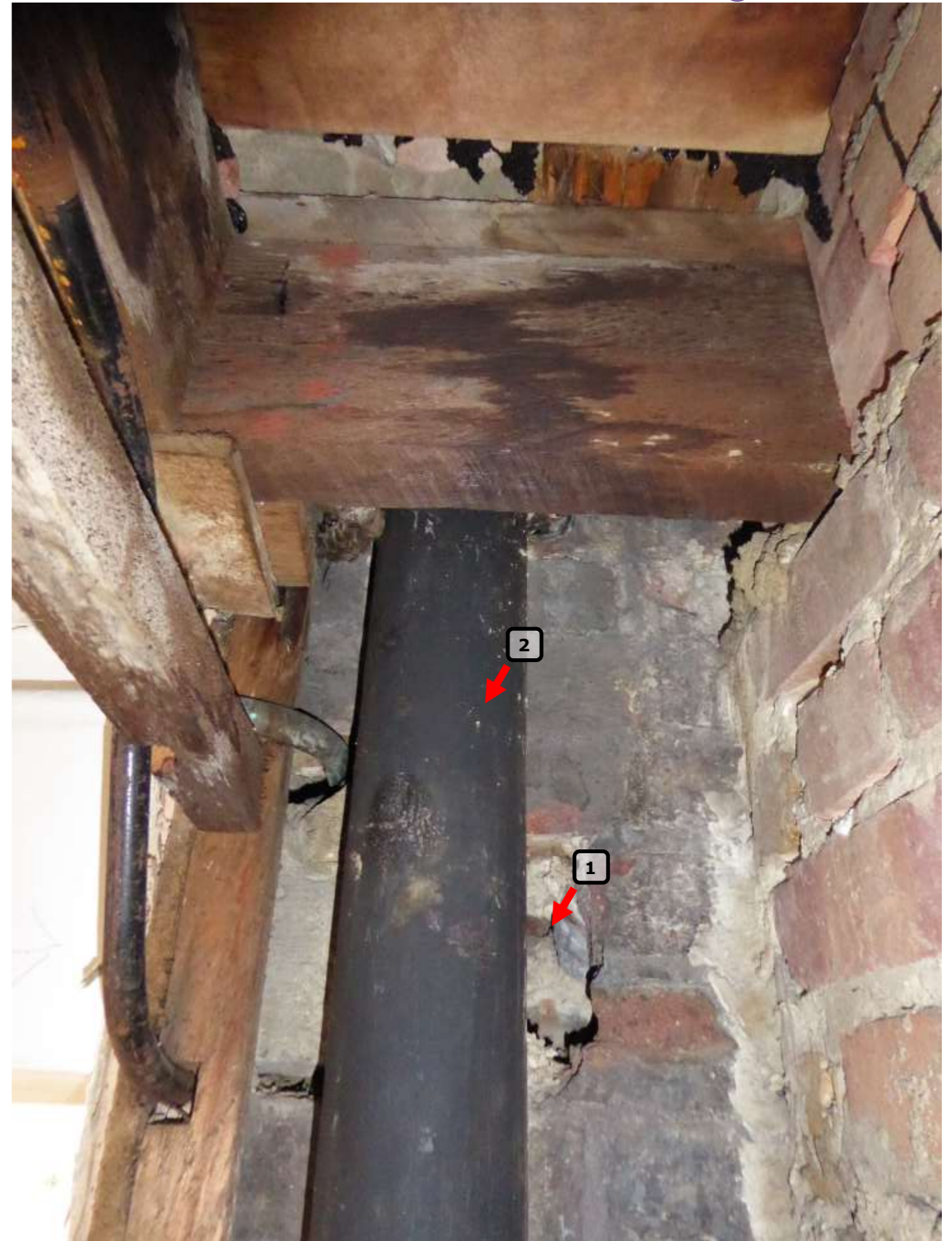
Plate FL2: The area that has been opened up. Note the down pipe [2] and the concrete lintel spanning the opening [1]. The down pipe can be seen externally at Plate E2 on page 15.
