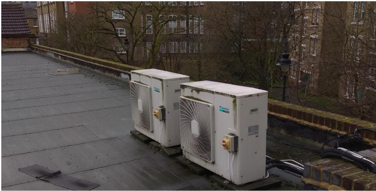
1. Location of AC units on main roof
