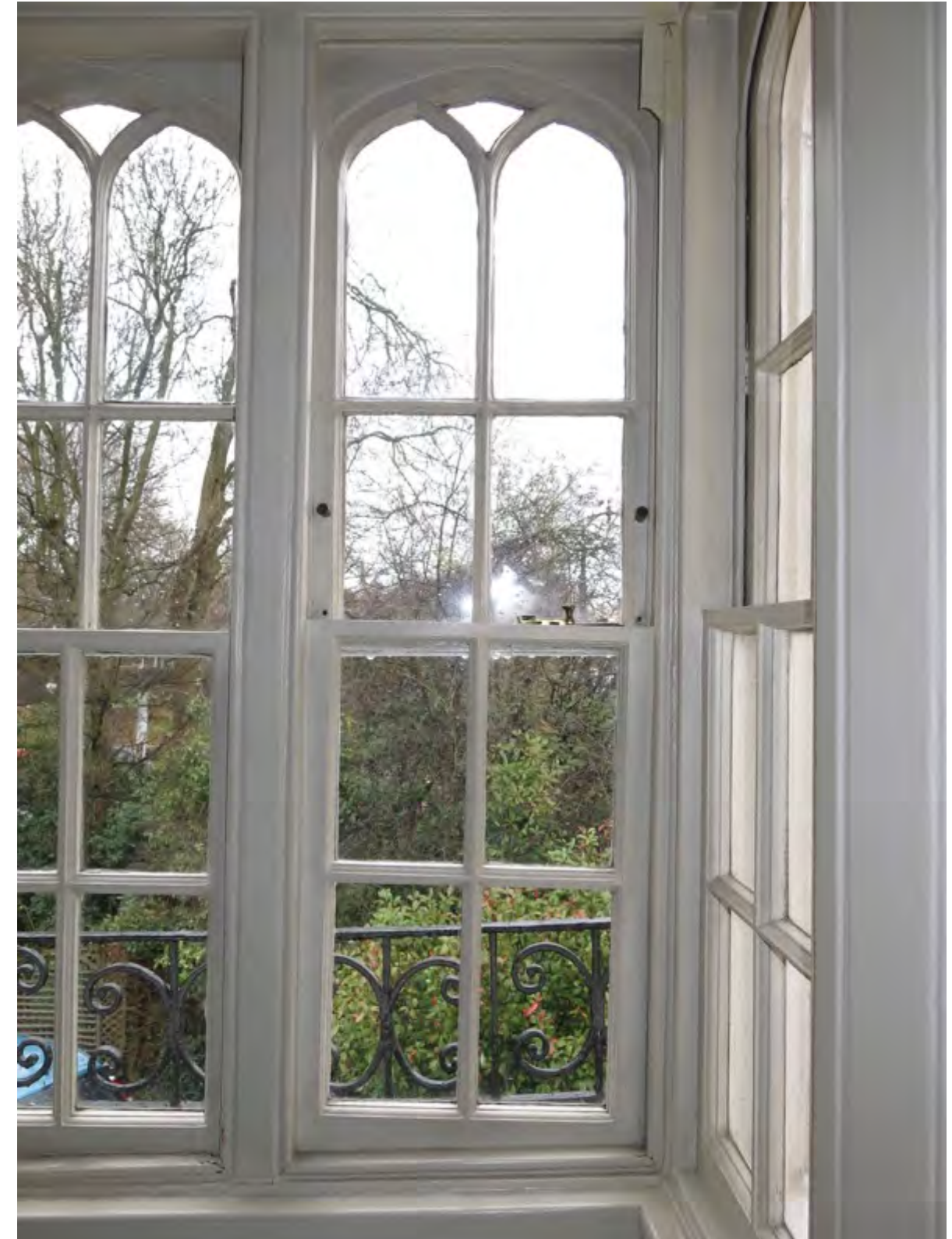
Figure 19: A detail of the existing sash windows. The existing window is distorted by building movement and has 30mm of horizontal misalignment
