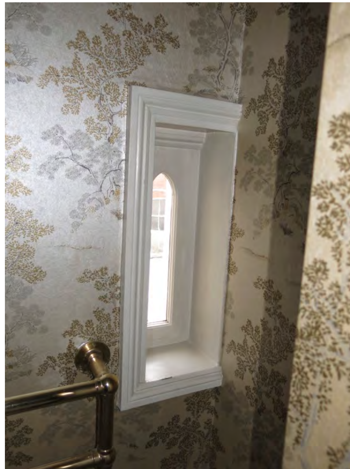
Figure 22: The right hand lancet window. Lift out secondary glazing unit will also be installed within this opening
