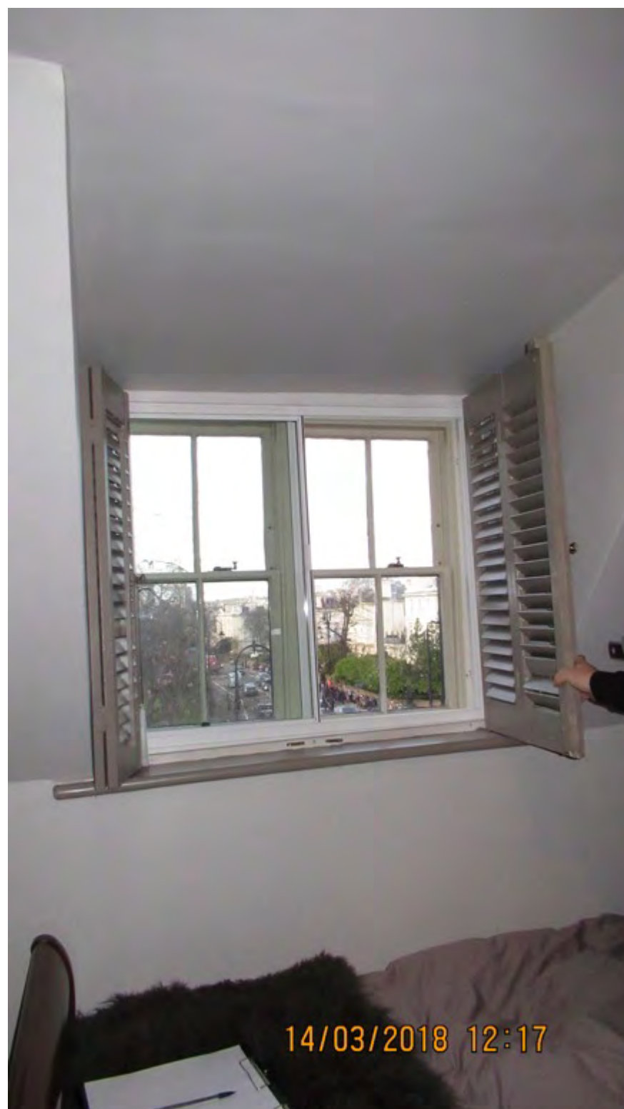
Figure 11: Internal view of the dormer window in the second floor bedroom facing north with existing secondary glazing installed. This secondary glazing will be replaced as part of the proposals
