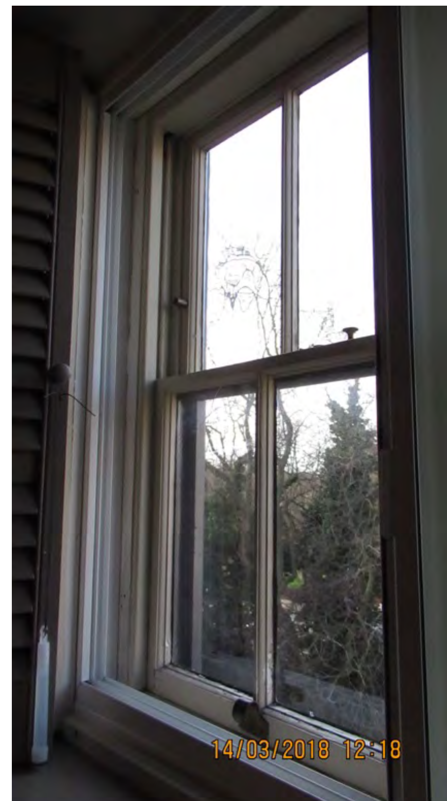
Figure 12: View showing the existing window jamb and cill illustrating the location of existing secondary glazing. The replacement secondary glazing will be installed within the jamb in a similar position maximising the gap between primary and secondary glazing.
