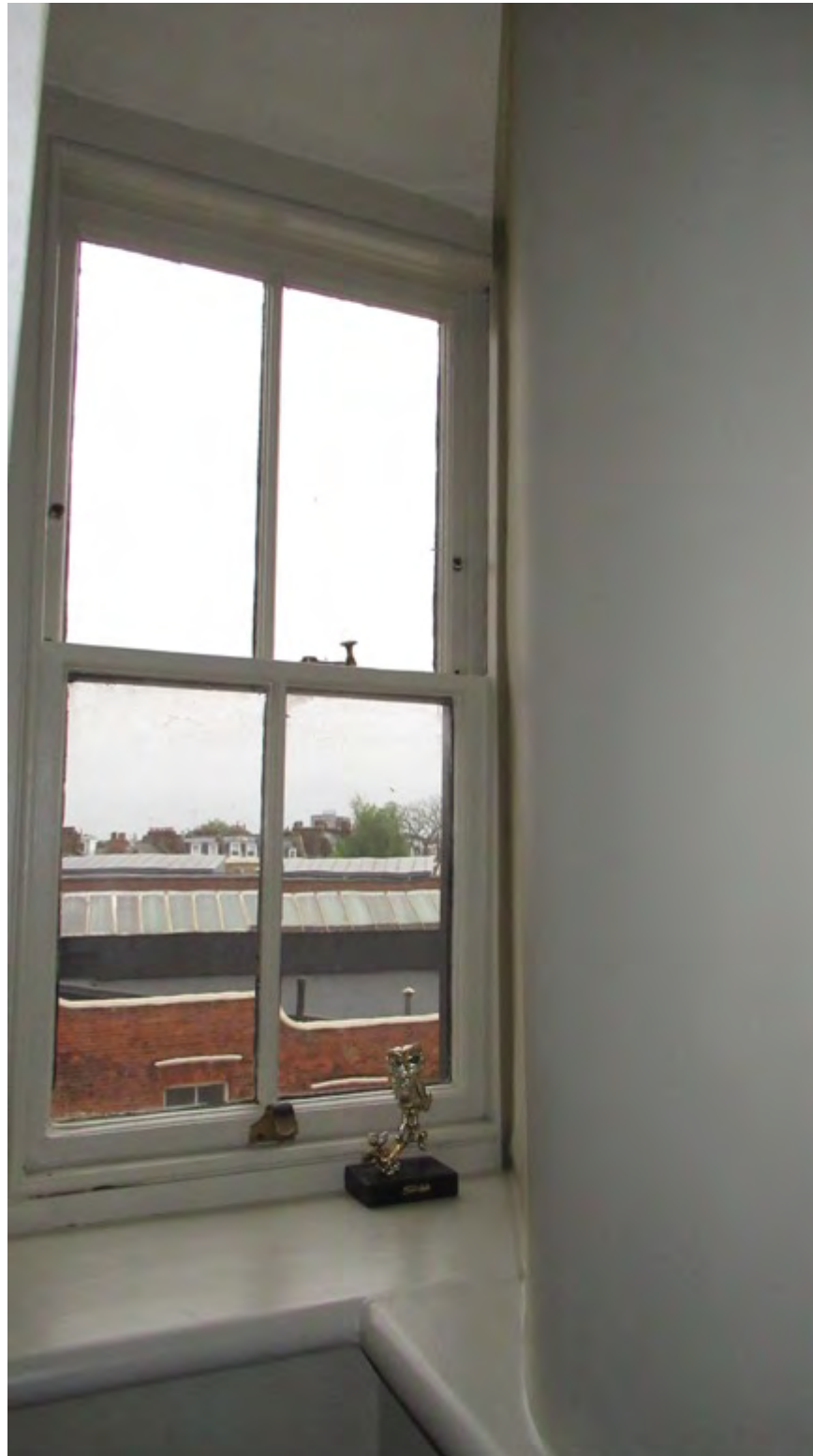
Figure 13: Internal view of the second floor landing window. The window is divided between the bathroom and landing by a stud wall. Secondary glazing will only be installed on the landing window
