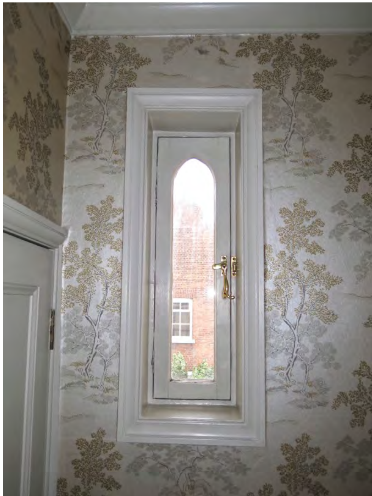
Figure 21: The left hand lancet window. A lift out secondary glazing unit will be installed within this opening
