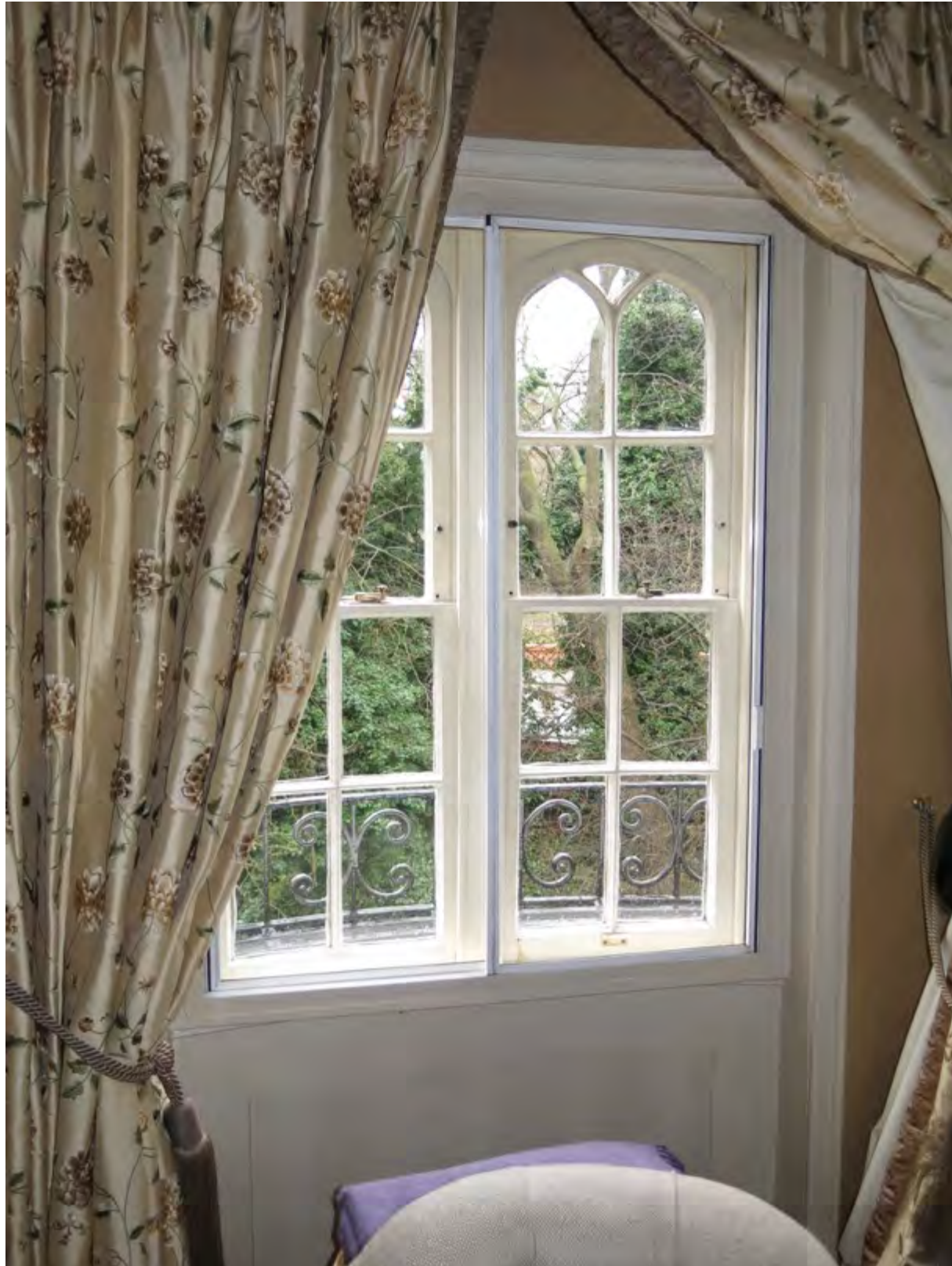
Figure 16: Internal view of one of the existing sash windows. All three windows are the same design and size. The new secondary glazing will be installed in the same position as the existing secondary glazing
