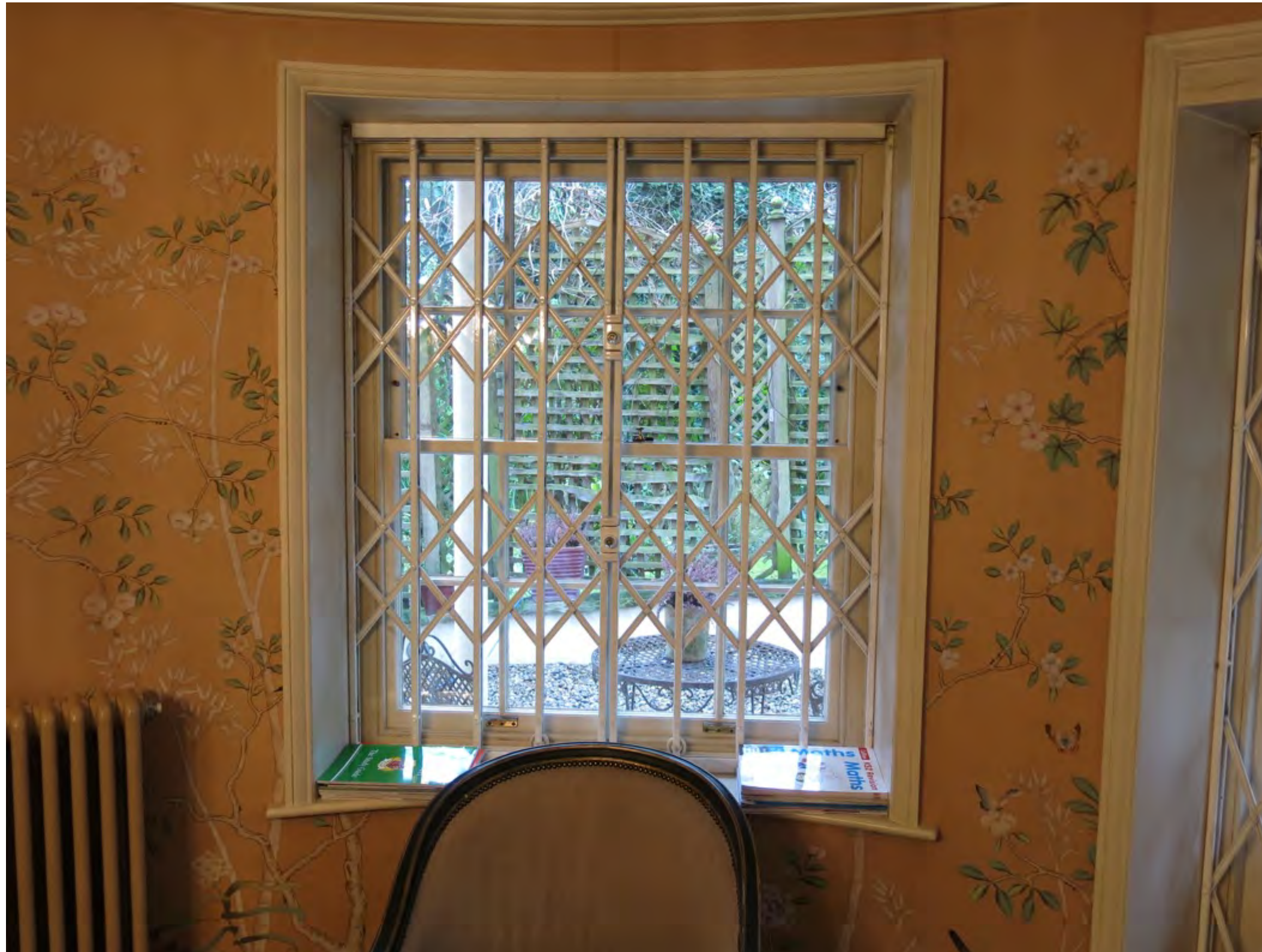
Figure 29: Typical sash window with existing security grills. Secondary glazing will be installed within the reveal in front of the security grill
