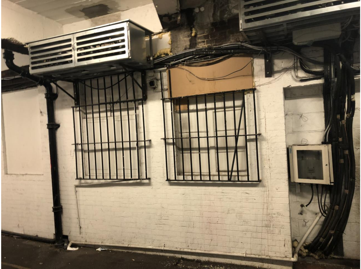
Alternative to connecting to existing ductwork – arrangement currently present to 4-6 Northways Parade, a wall mounted exhaust unit
