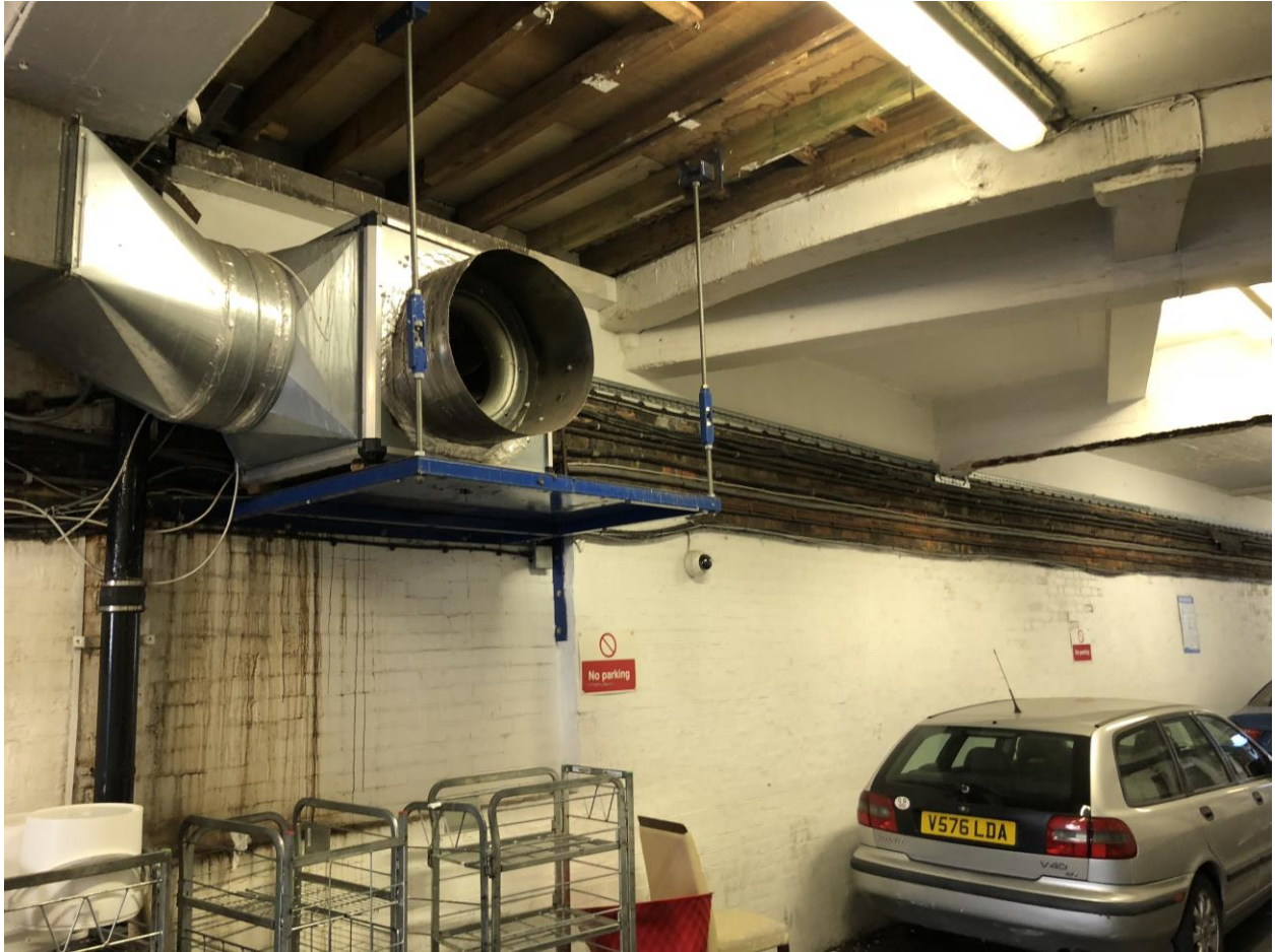
Existing Ductwork that may be connected into
