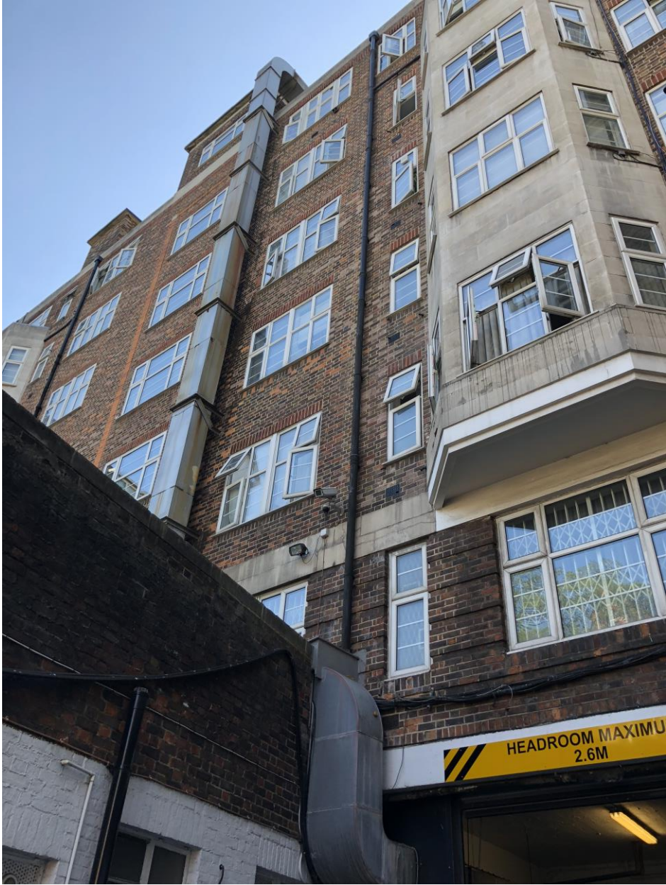
Ductwork route up side of building
