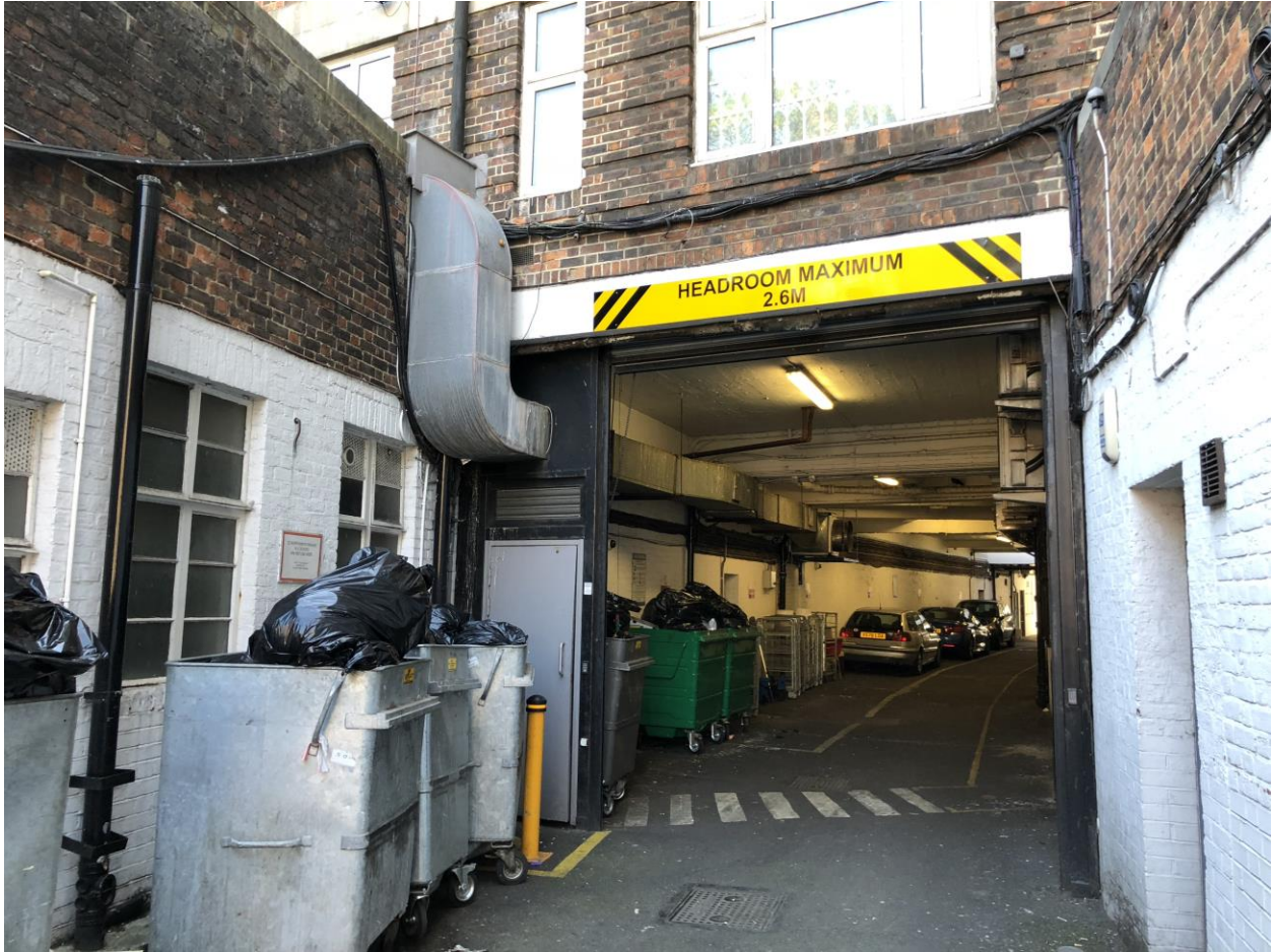
Ductwork route out of service road
