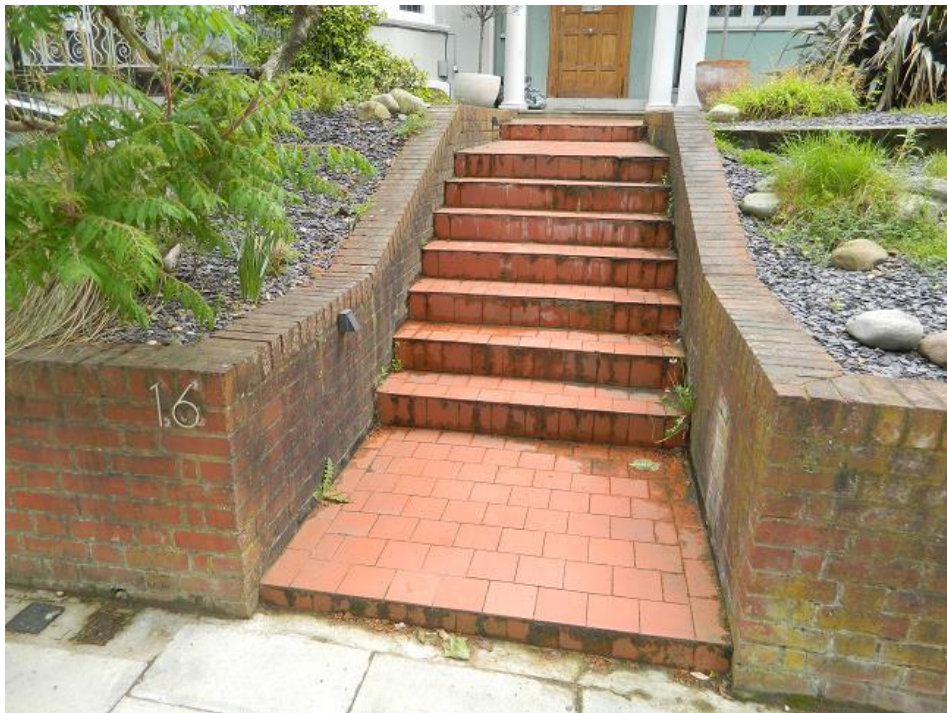
Figure 4. Photographs showing retaining walls and steps at the front of the property.
