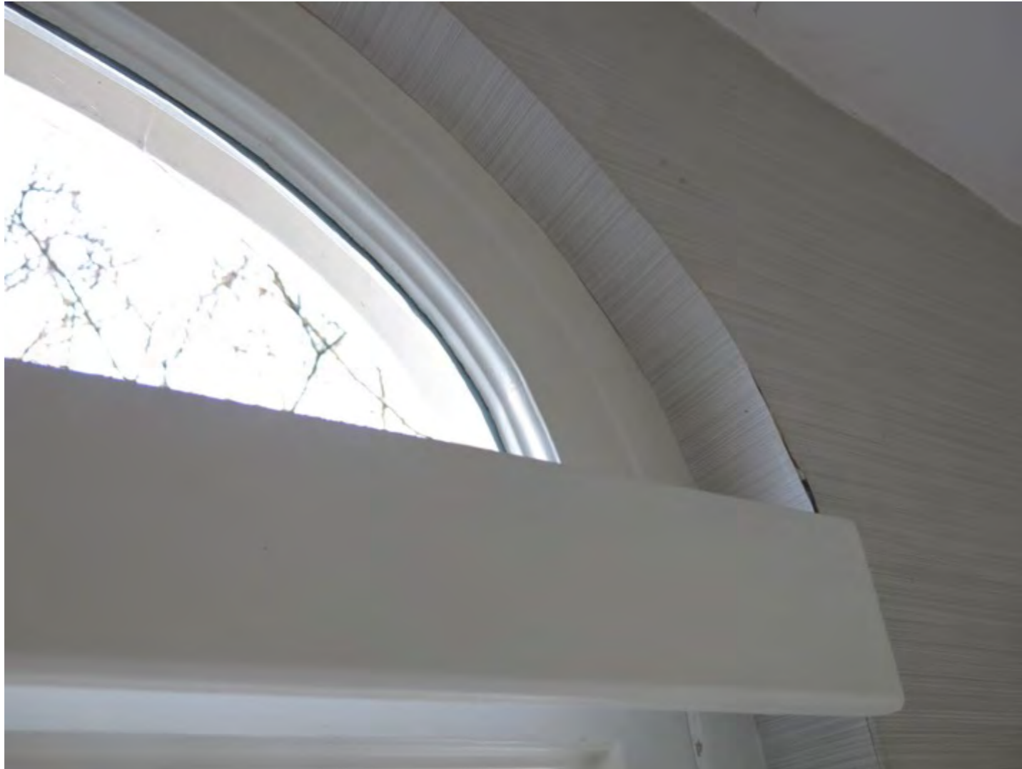
Figure 20: Detail of the existing curved window head (a three centred arch) with existing blind box
