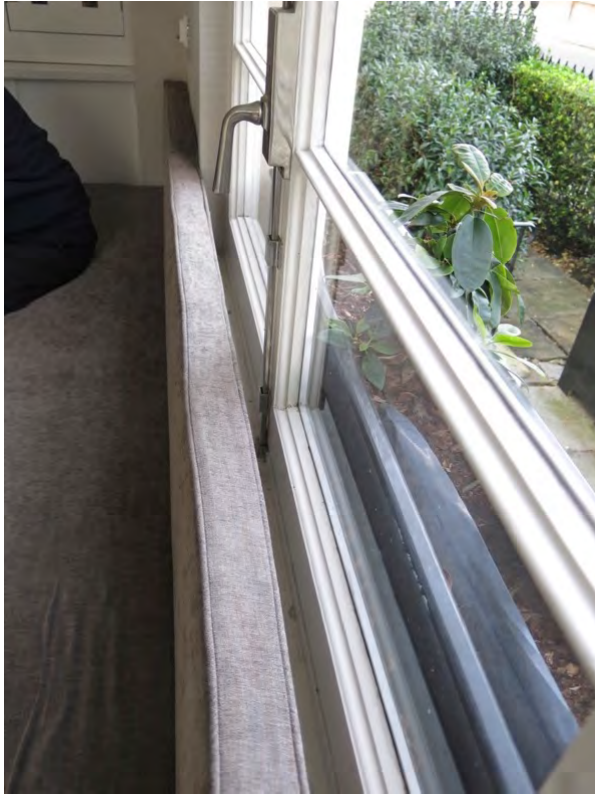
Figure 18: Existing window seat back (secured by Velcro) will be move forwards by 50mm and secured to the face of the new secondary glazing
