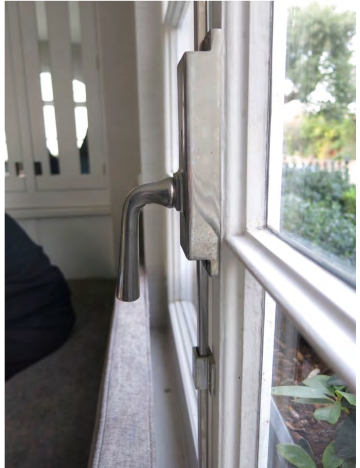
Figure 17: Detail of the modern window which replicates original windows. The espagnolette lock handle will be temporarily removed to allow the secondary glazing to be installed but can be refitted (push fit and secured with recessed 'grub screw') by the resident to open the existing windows
