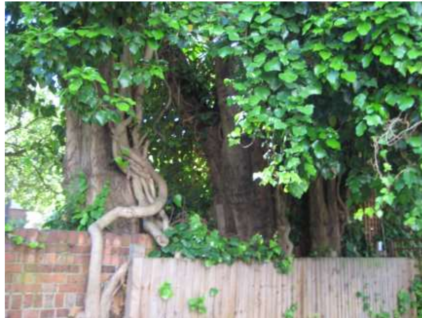
Fig 1 – There are very large Ivy stems on the lower trunks of TG1 and given the tree sizes and locations we would advise this is severed to allow better future inspections.
