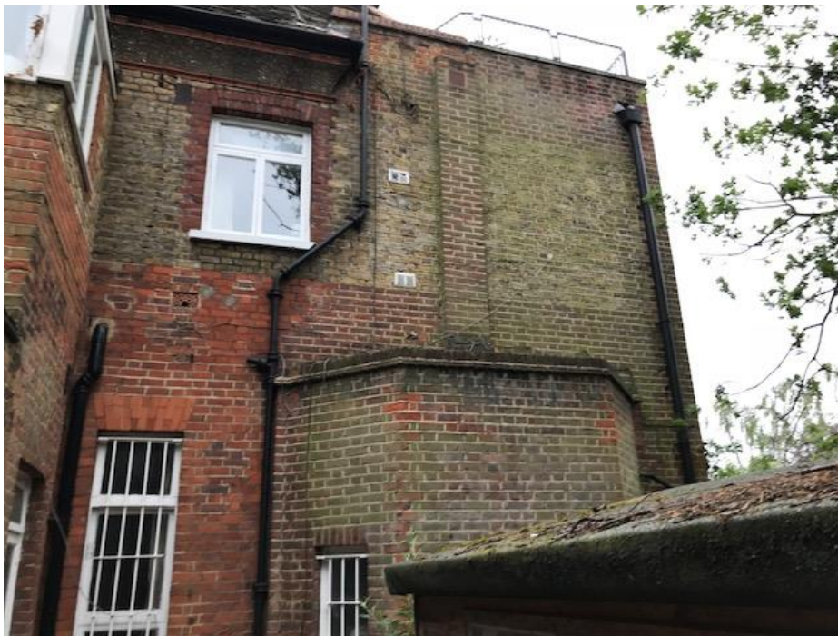
2. Rear elevation (Note bay window and outbuilding to be replaced by proposals)
