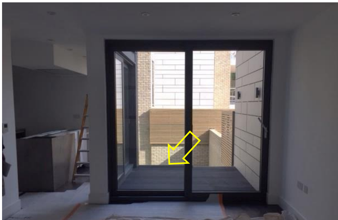
Photo.1 View from within No.18 looking out over terrace towards the garden. Arrow indicates extent of proposed extension.
