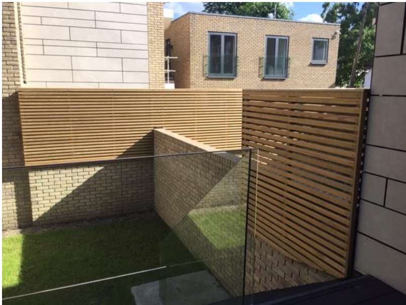
Photo.3 View from terrace showing mixed block (under construction) and the Studio apartments.
