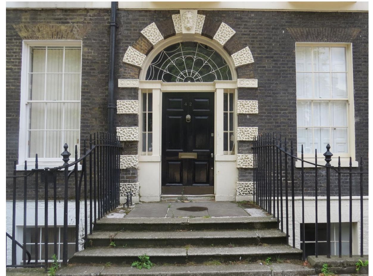
Fig. 3. Photograph showing the main entrance to 42 Bedford Square, prior to works commencing.
