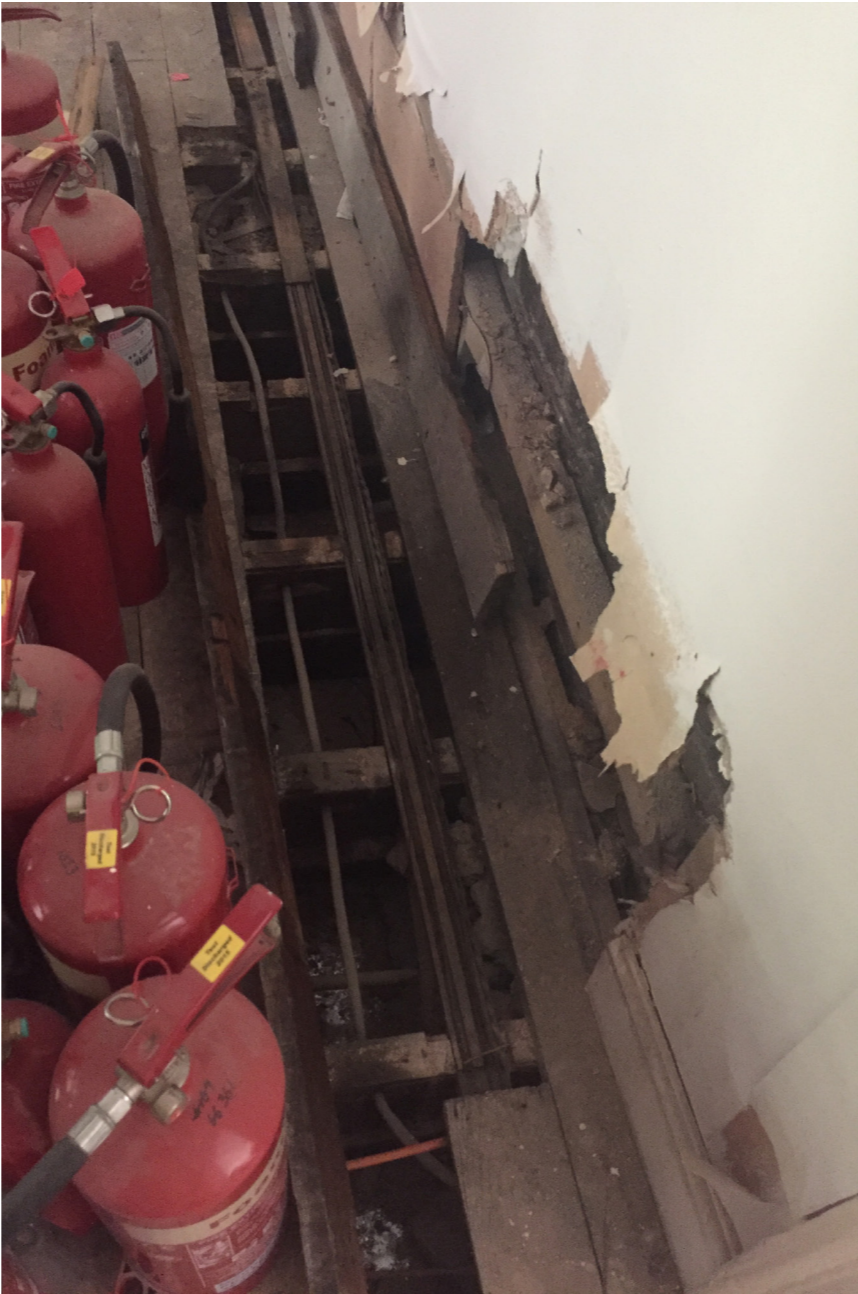
Picture 2 - Ground floor. Existing notching.
