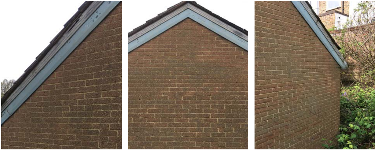
No evidence of significant cracking, damage or deterioration of brickwork. Wall is in relatively good condition with no visible cracks and is marked for protection, propping and retention.
