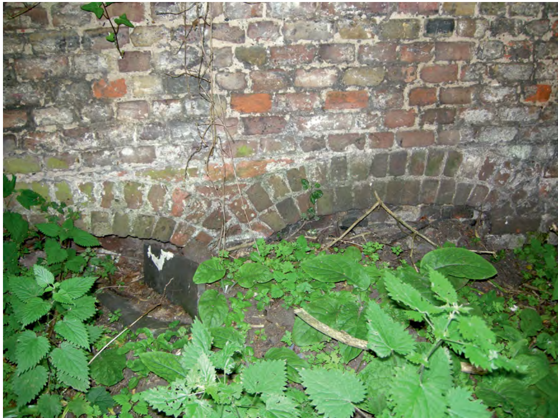
Fig 16 Bottom of north-east wall of store along south-west wall of 6 Streatley Place; view looking south-west (MOLA Photo 16.06.2014)
