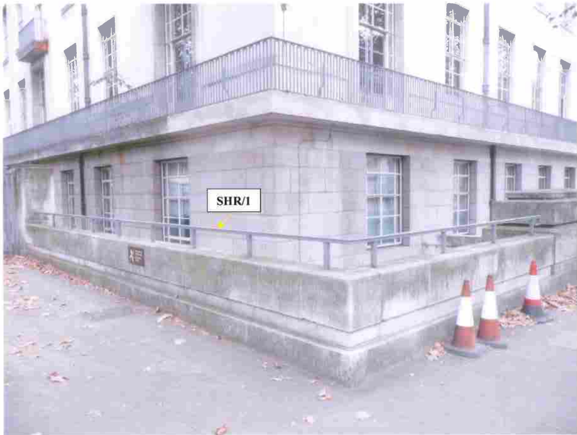
Low Guard Rail on SW corner of the building (Malet Street and Montague Place) (see sample SHR/1 in Appendix Two)
