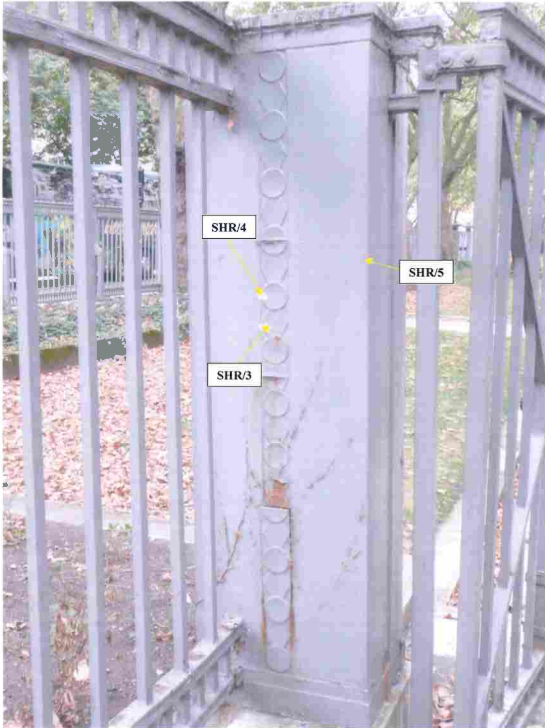
Gate Pier SW Corner. Note the Decorative Detail (see samples SHR/3; SHR/4 and SHR/5 in Appendix Two)
